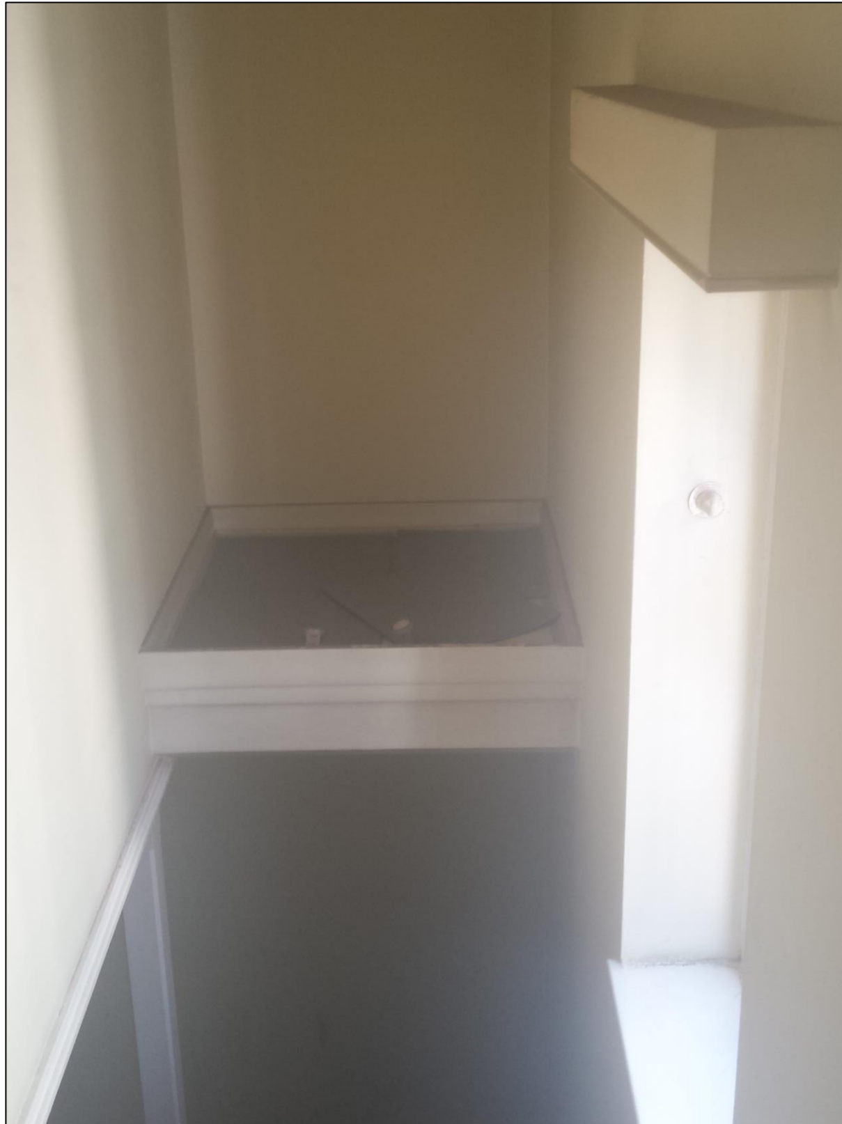
Figure 10 Stairwell area between third and fourth floor - proposed to be boxed in and extended into the adjacent bathroom.
