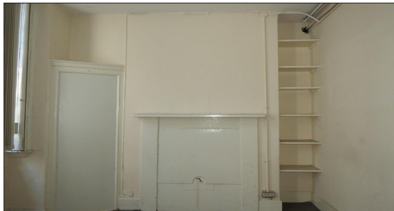
Figure 4.12: Interior of a room at second floor level in the front part of the building
