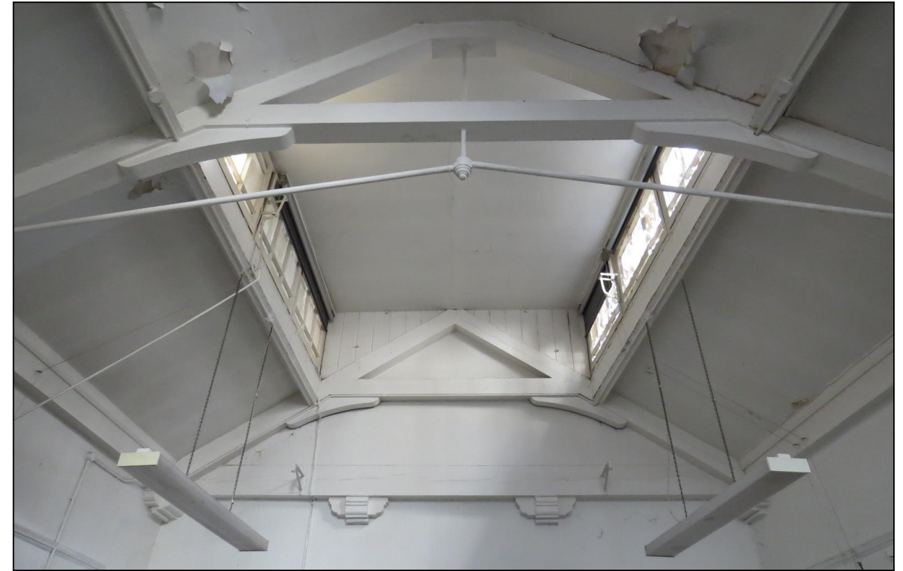
Figure 4.9: Roof to the possible chapel to the rear of the ground floor
