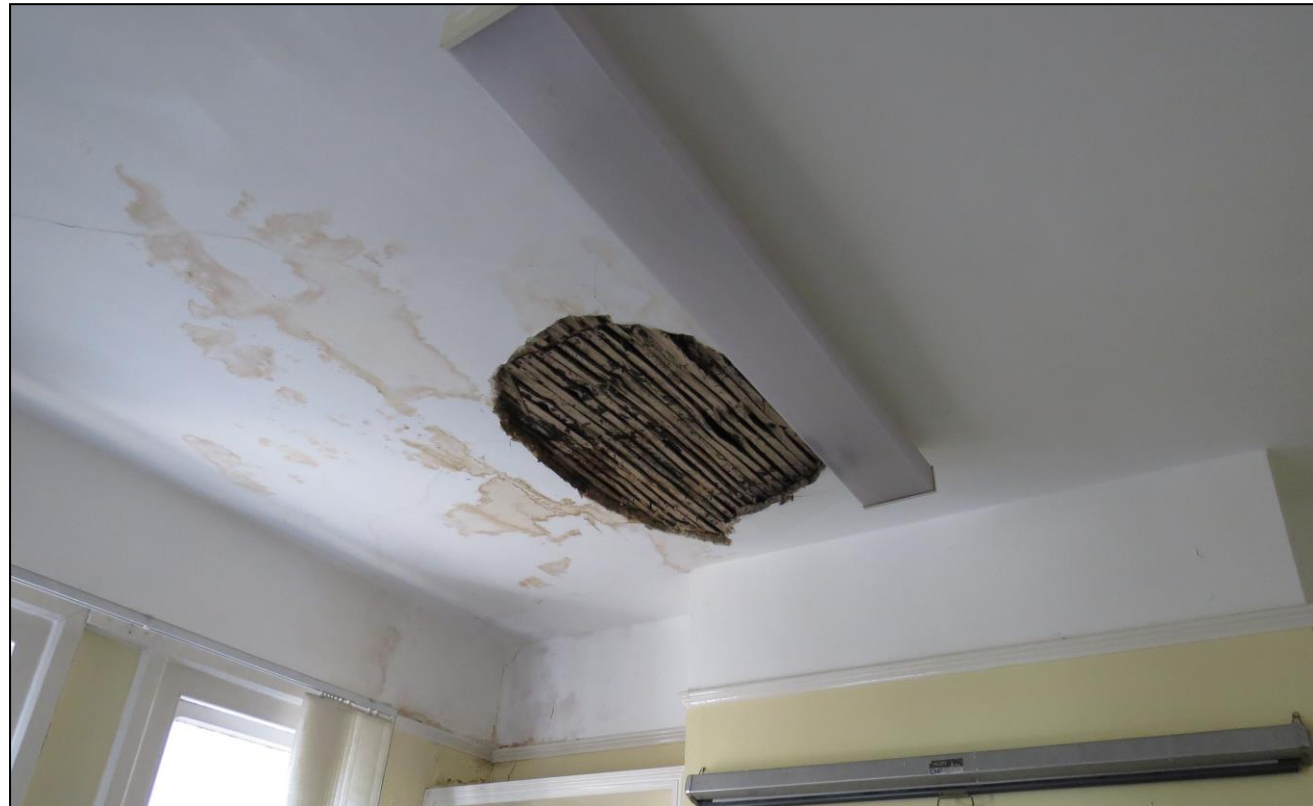
Figure 4.11: Lath and plaster ceiling exposed by local ceiling collapse, likely to be original
