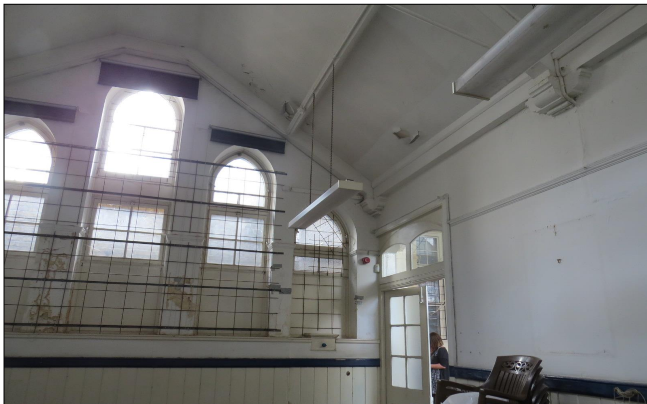
Figure 4.8: The possible chapel to the rear ground floor, showing fenestration in west elevation
