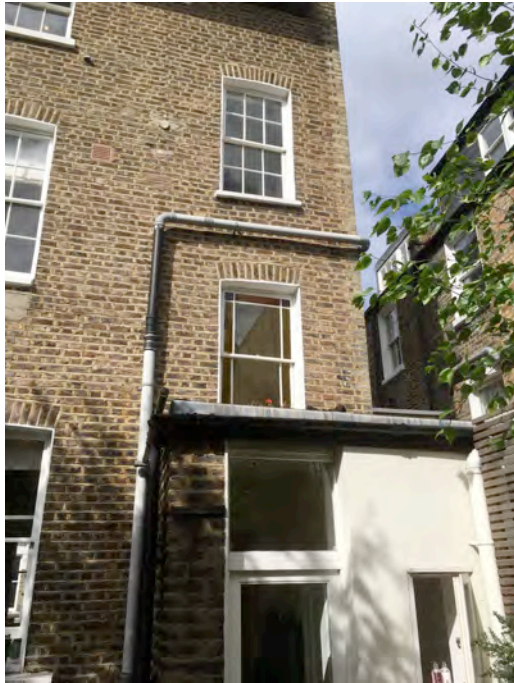
Rear elevation- closet wing showing rear door and WC window, proposed extension location
