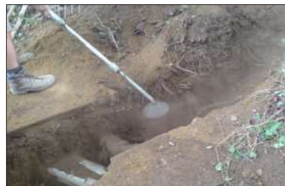
Excavation image 2: Air spades are very effective at exposing roots and services with minimal damage.
