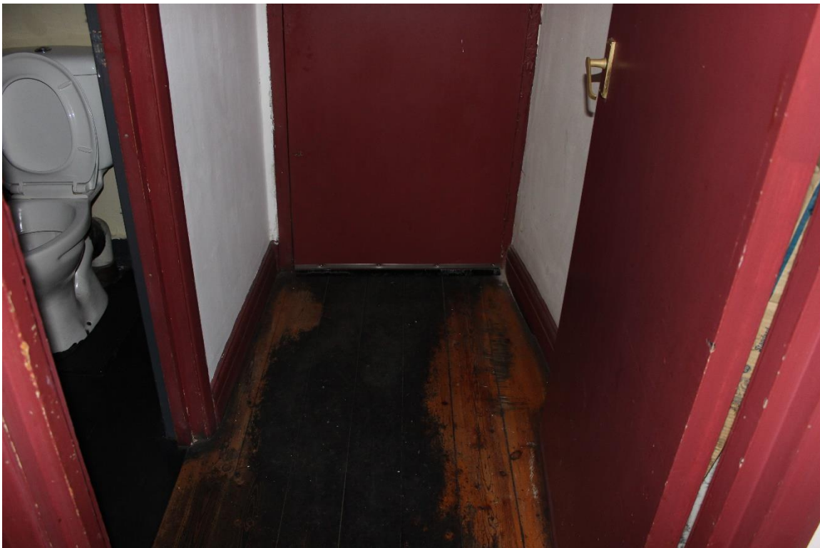
238 West End Lane – Existing WC viewed from the entrance to the kitchen
