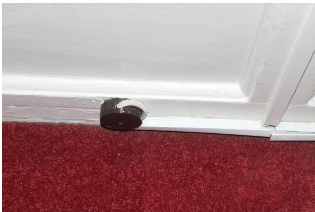
47. Poor electrical detailing.
