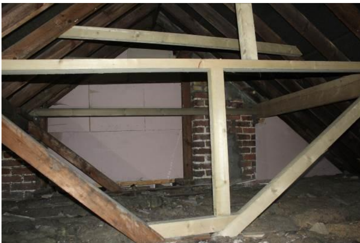
33. Additional roof supports and fireproofing of party wall to main roof space.
