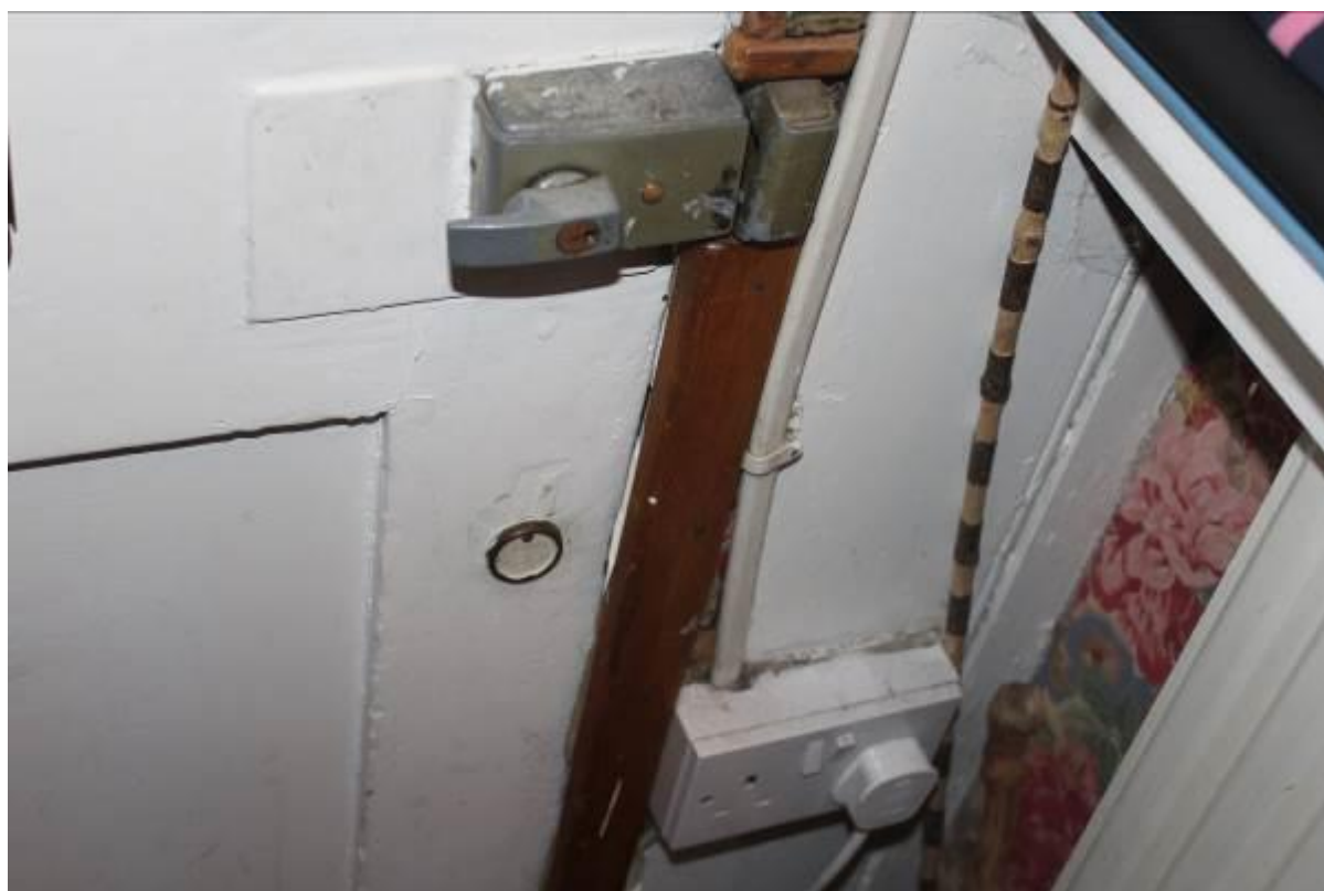
43. Air gap between door and frame.
