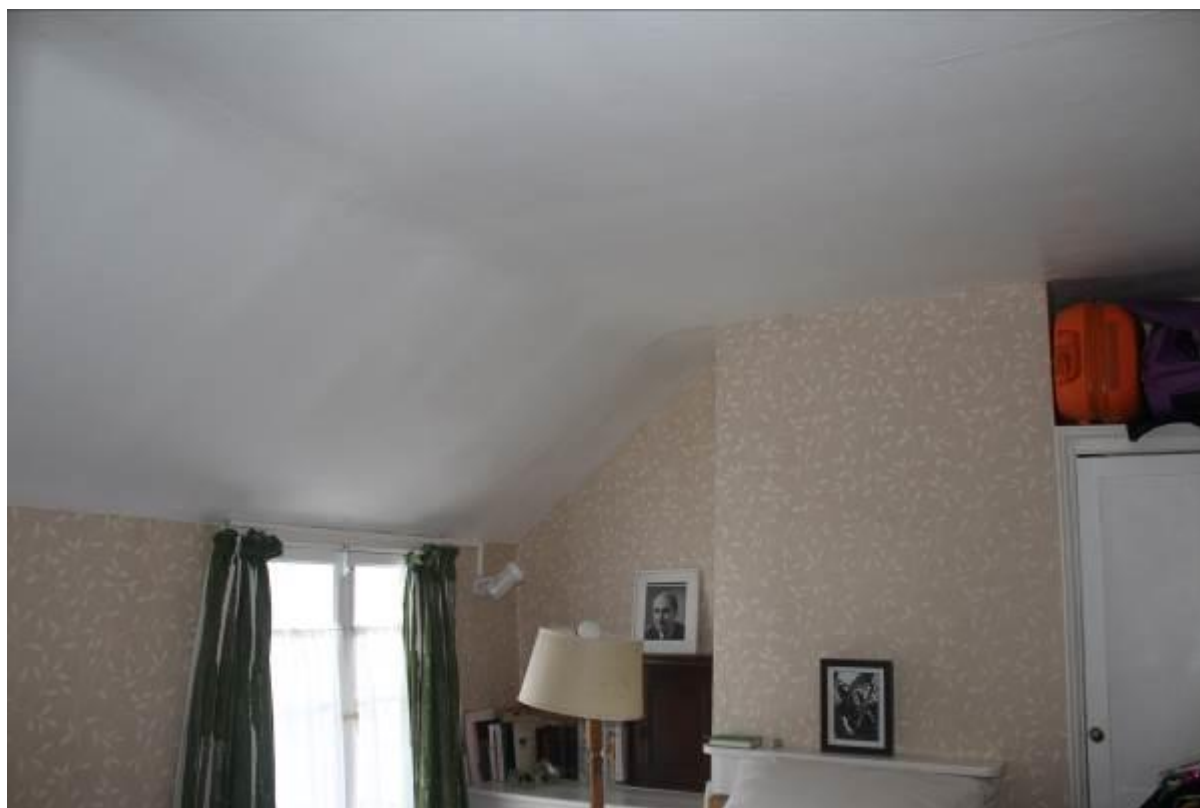
38. The roof construction has caused the rear wall to spread as demonstrated in photograph 12, but there is no significant evidence of this being ongoing.
