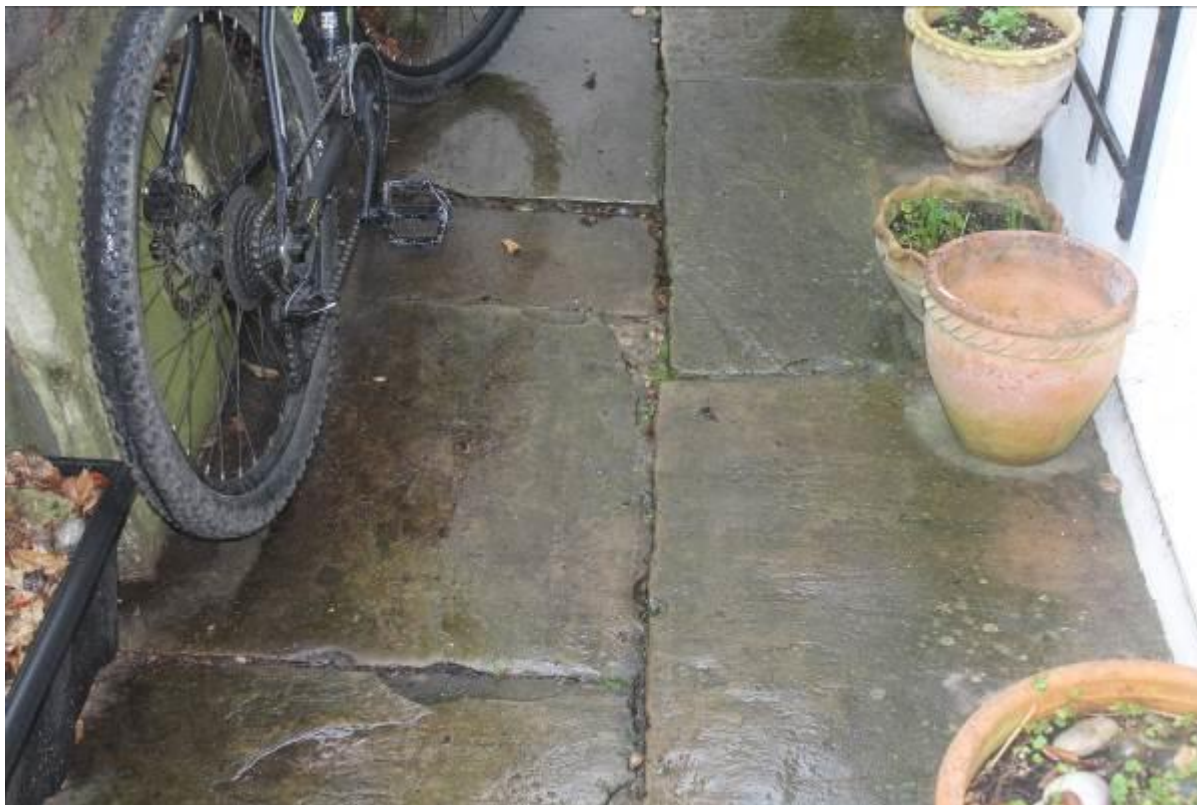
13. Rainwater percolates through the paving gaps causing them to settle unevenly and contributes to the movement to the flank wall, this is why we recommend a damp membrane is located under these slabs.
