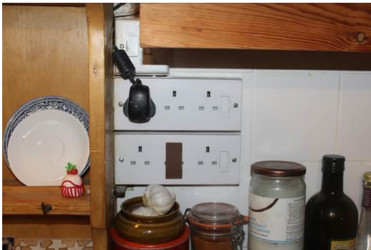
46. Poorly designed electrical socket facilities, also note one of the positions has been blanked off with tape. Further investigation or rewiring required.
