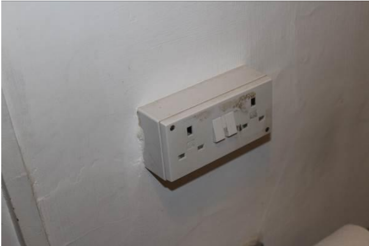
50. Socket outlet in cloakroom contravenes the IEE wiring regulations.
