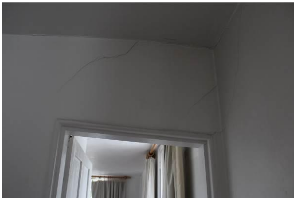
39. Slight cracking above first floor door opening indicating movement is ongoing.
