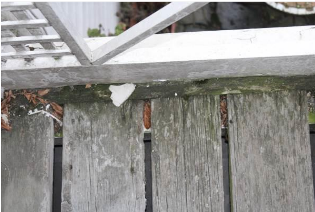
19. Ends of balcony decking showing signs of decay.
