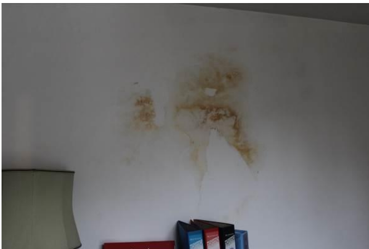
24. Plaster repairs required to first floor bedroom where water damage has occurred.
