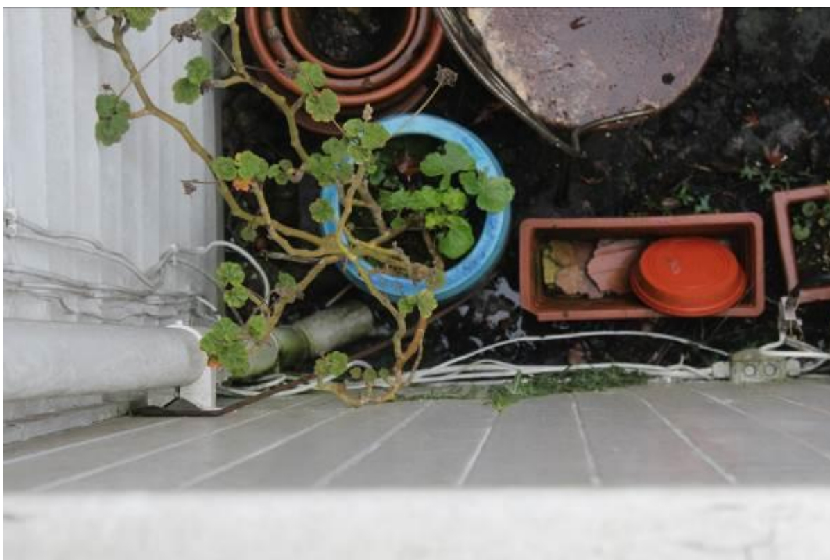
20. Rainwater build up noted in adjoining property to downpipe serving west elevation roof. Further investigation and repair/unblocking is required.
