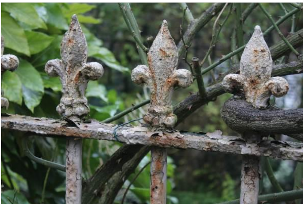
8. Redecoration required in conjunction with careful removal of corrosion to boundary railings.
