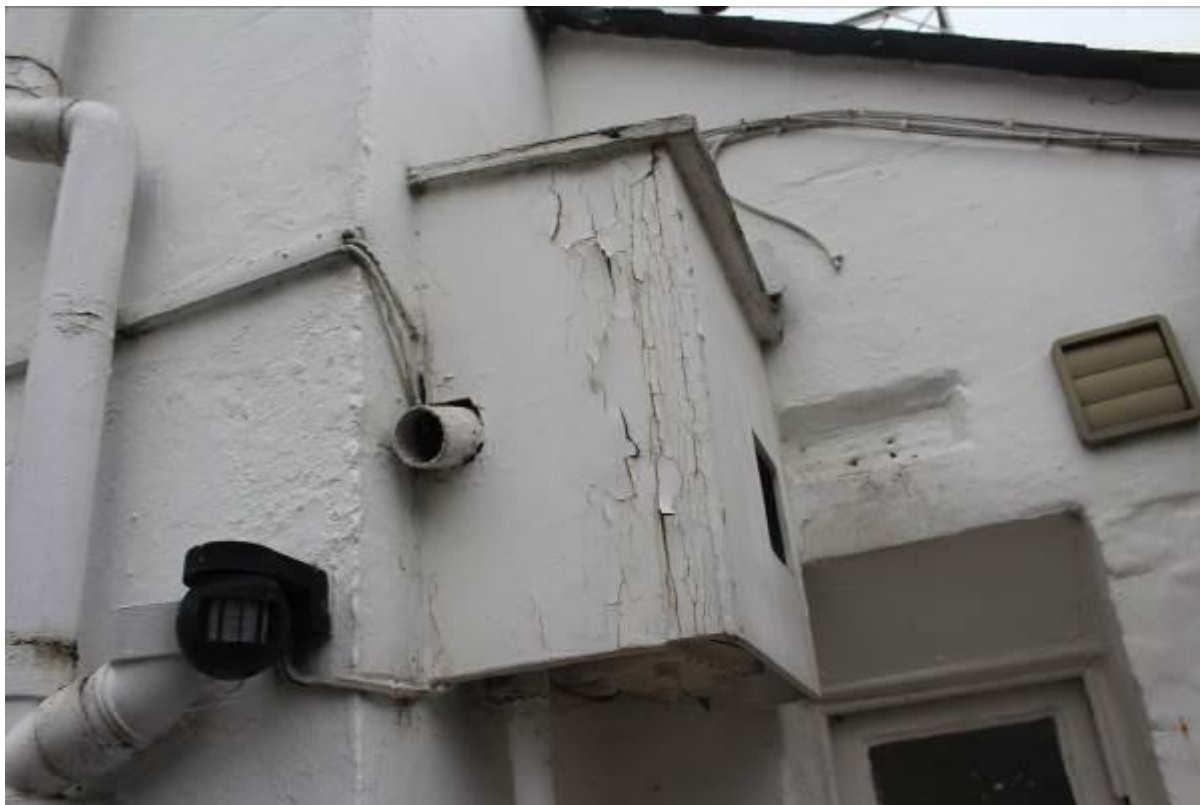
26. Repair and redecoration of gas meter box is required.
