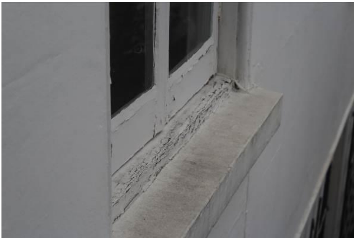
21. Redecoration and repair required to external joinery to rear addition.
