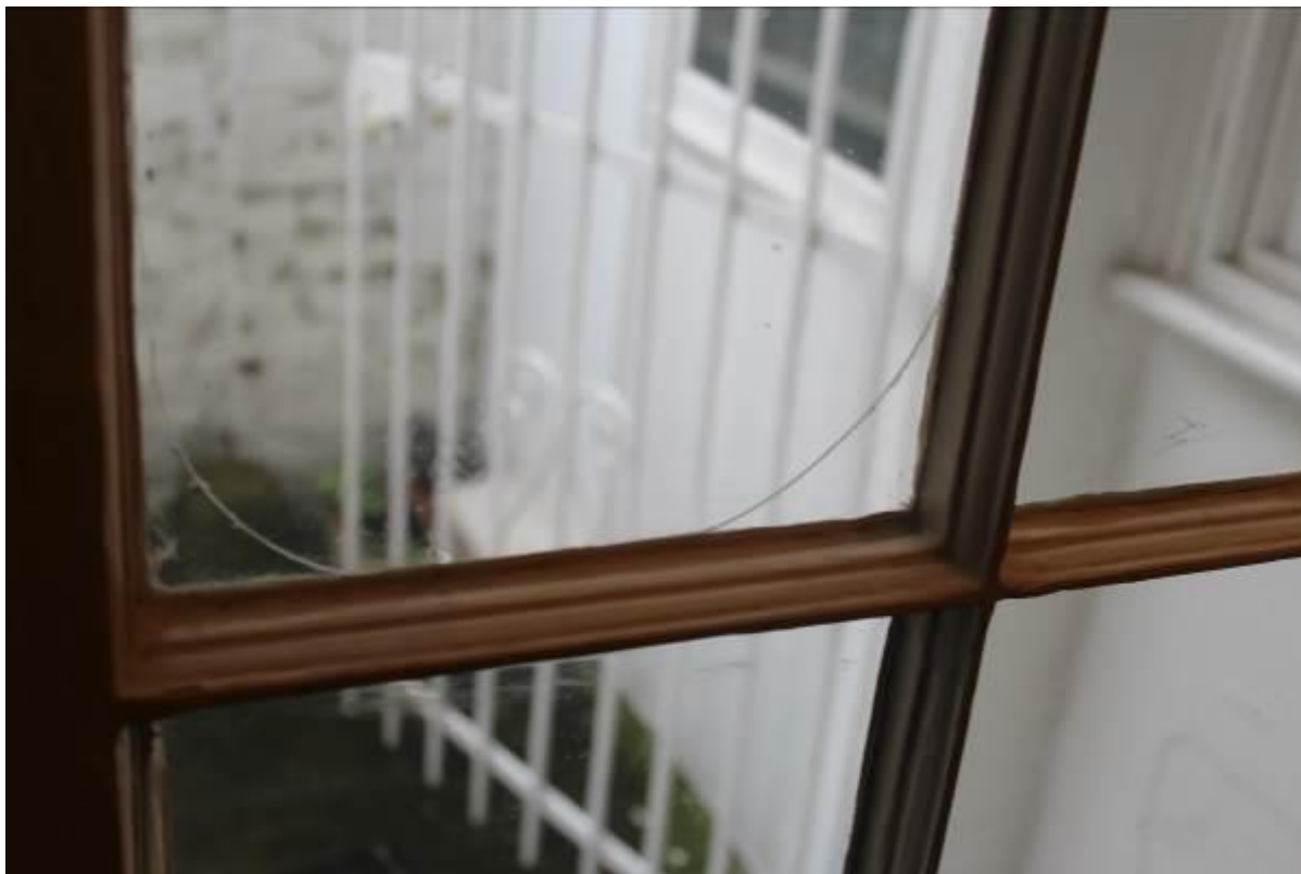
44. Replace broken glass pane.
