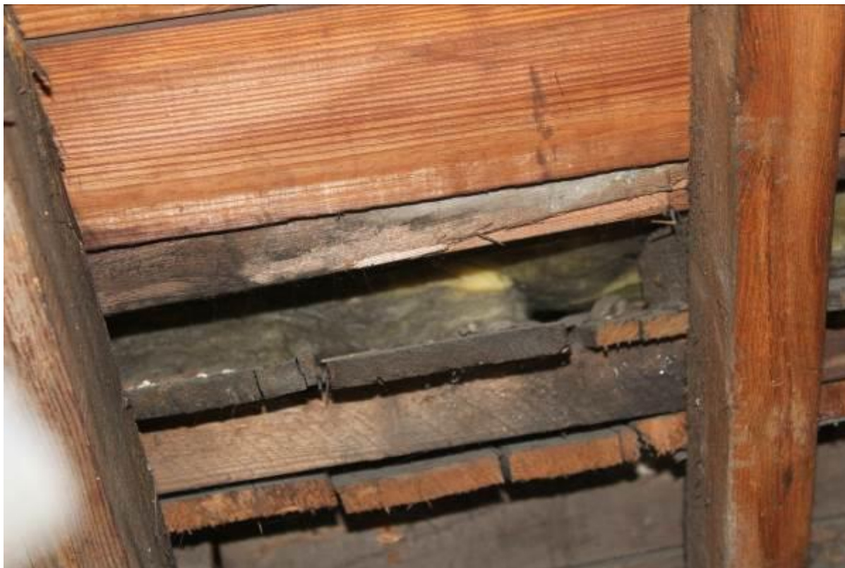
32. Evidence of some insulation in back addition roof space as viewed from the front roof space. An access hatch in this roof space is recommended.
