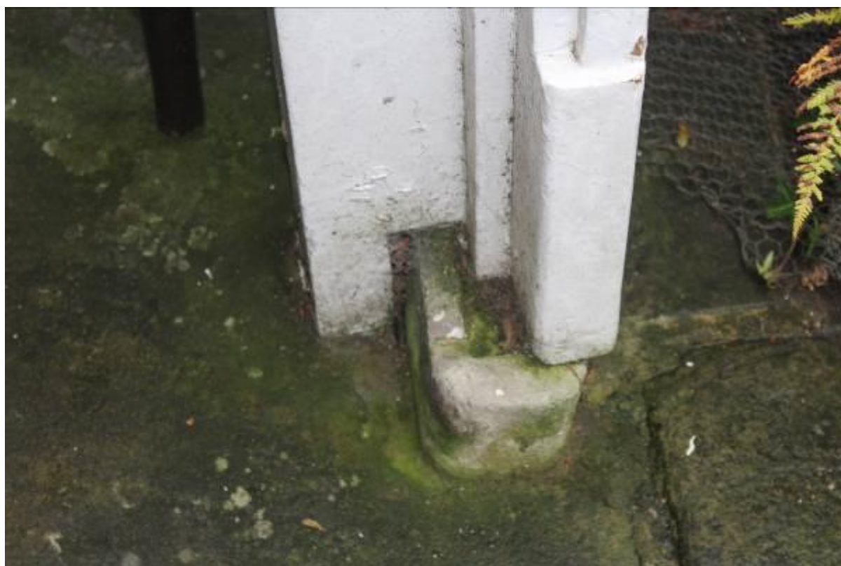
29. Front balcony support base now out of alignment and in need of re-seating.
