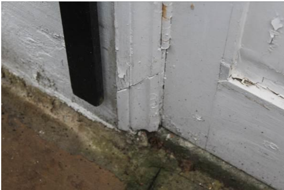
17. Poor internal quality architrave timber used, this should all be redtailed.
