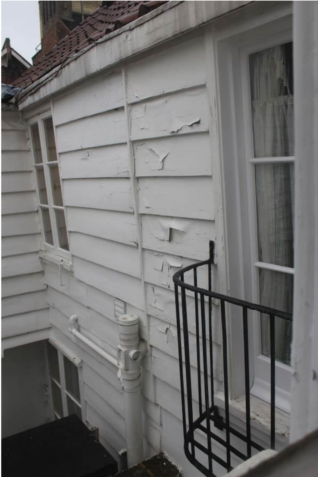
12. Deviation in the external rear wall caused as a result of roof spread.
