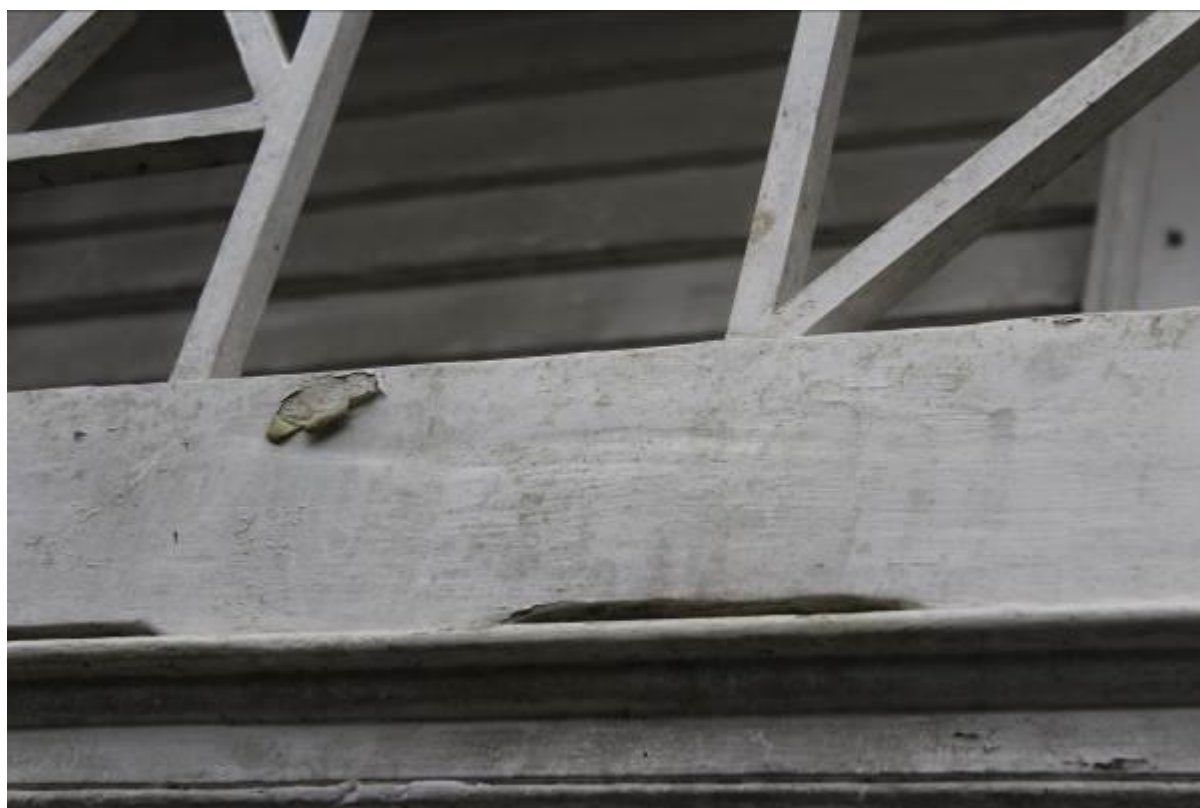
4. Timber decay evident to balcony structure.
