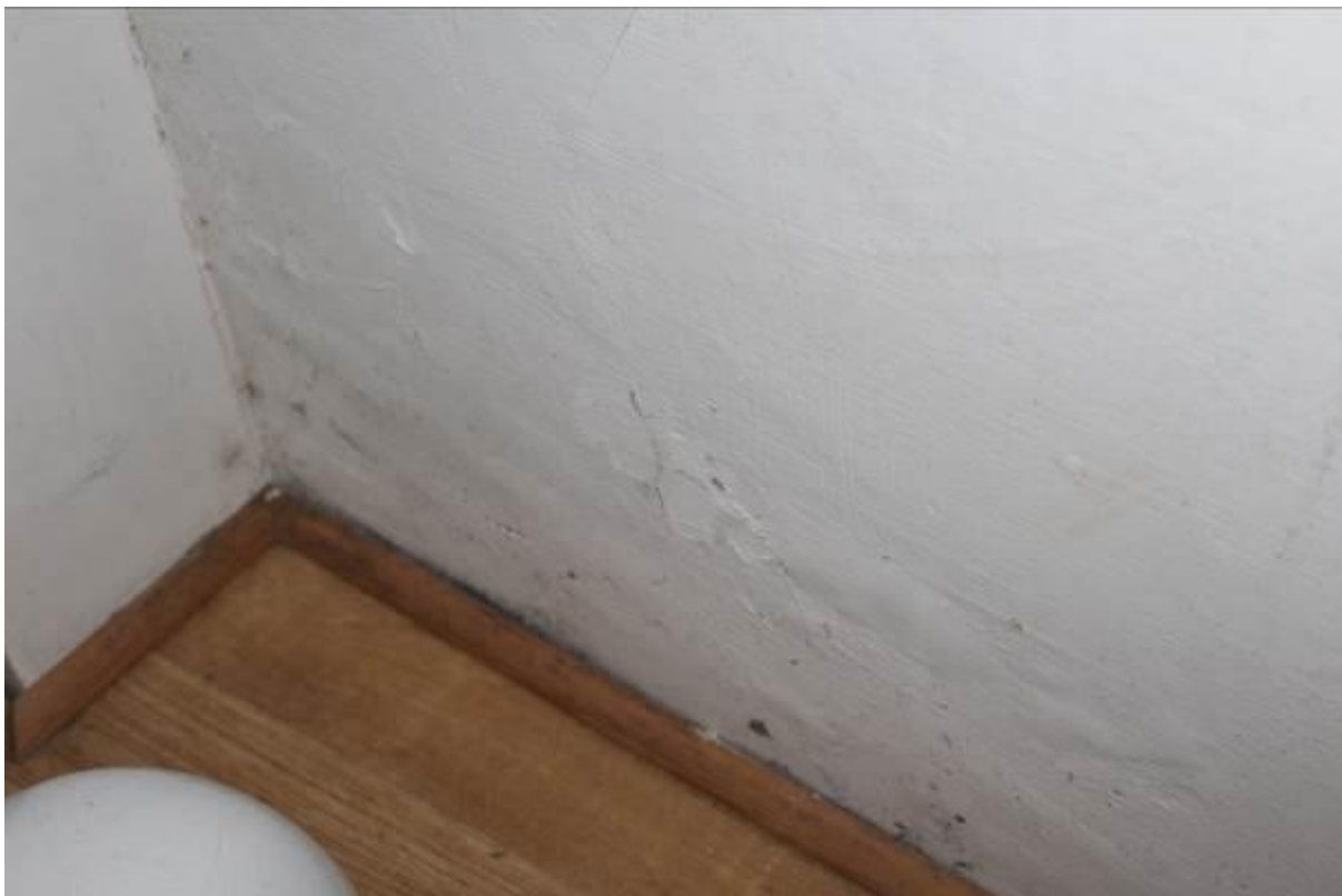
41. High damp readings noted.
