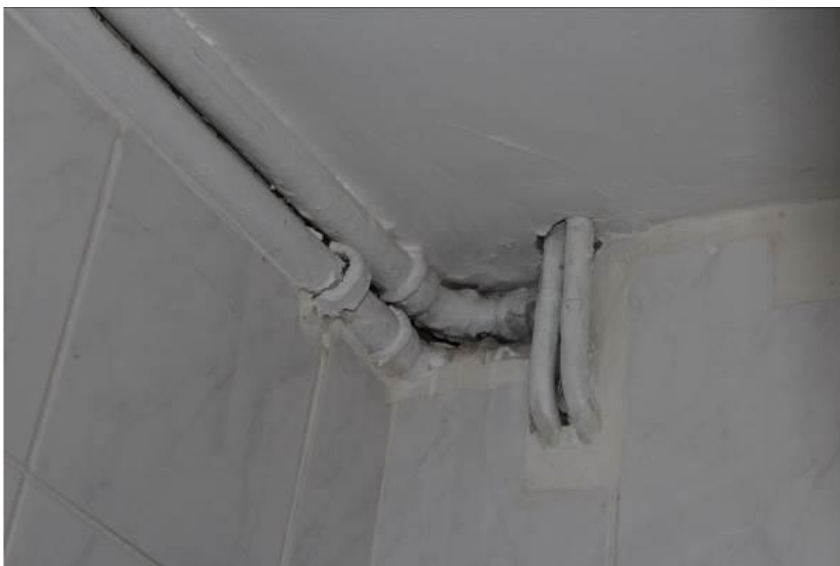
45. Surface run ground floor pipework, unsightly, recommend concealment if not redundant.
