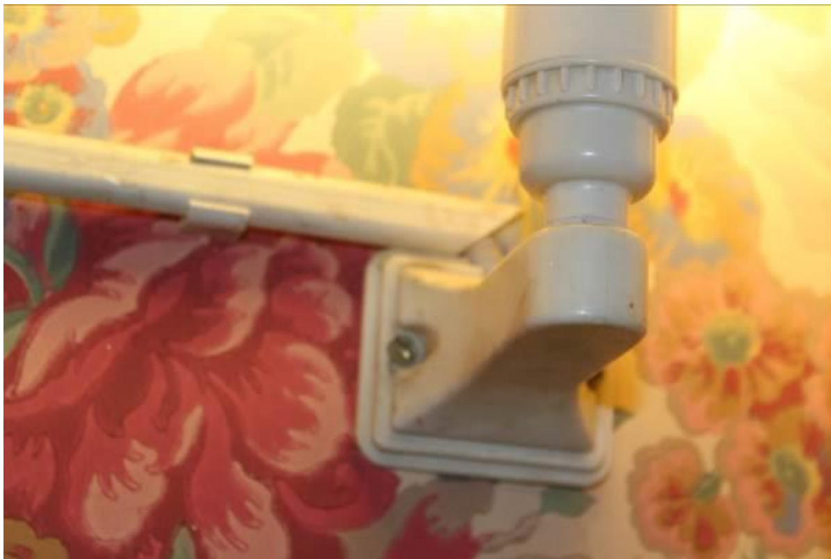
23. Poorly formed surface run conduit.
