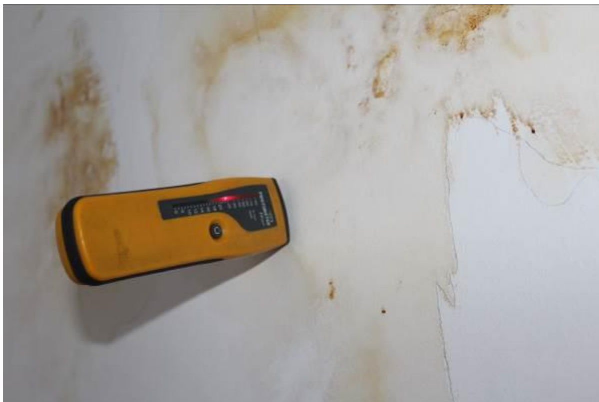
42. High reading noted in first floor bedroom, this could be caused by salt contamination, replastering required and further investigate by inspecting roof above.
