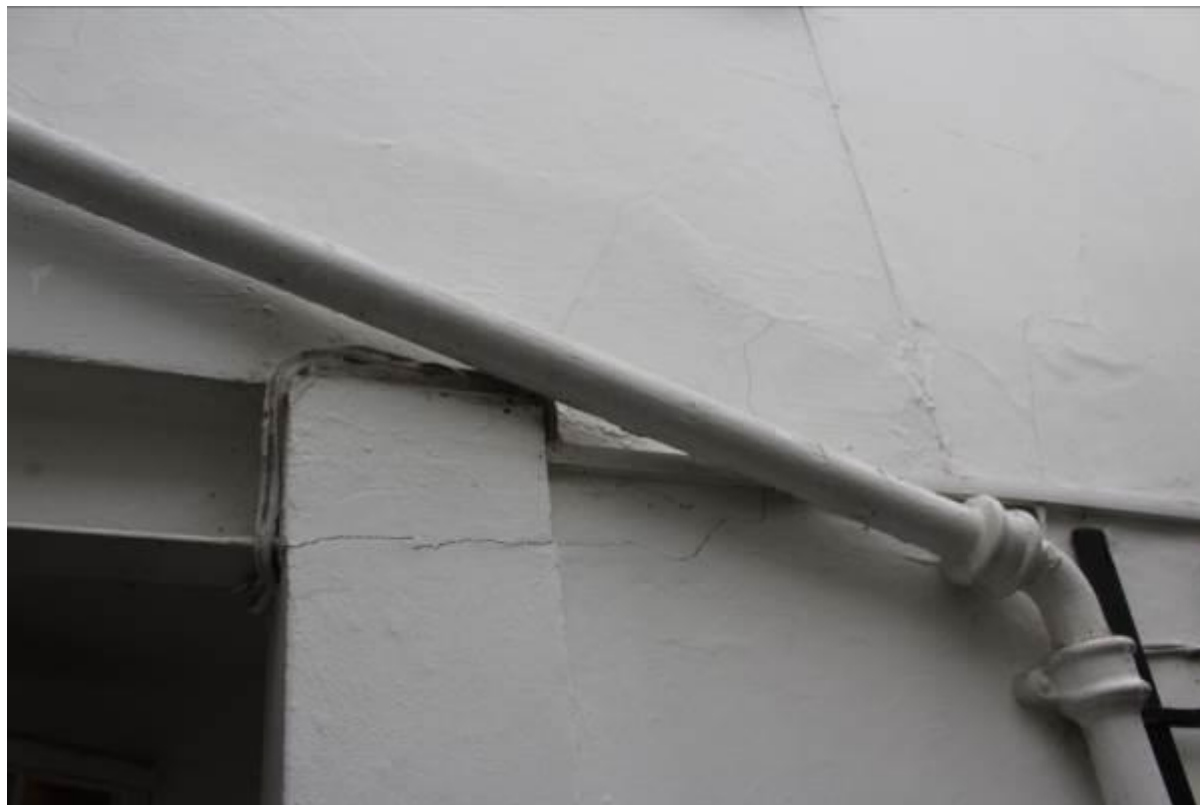
28. Some cracking observed to rear addition masonry indicating the movement is slowly ongoing.
