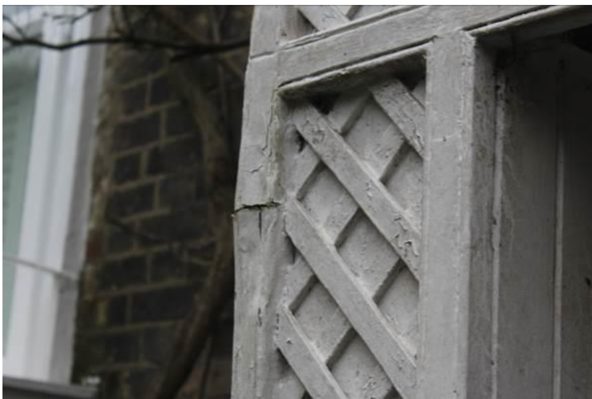
6. Window care repair required.
