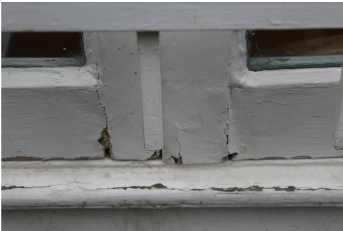
15. Joinery window care repairs required to some rear addition windows.
