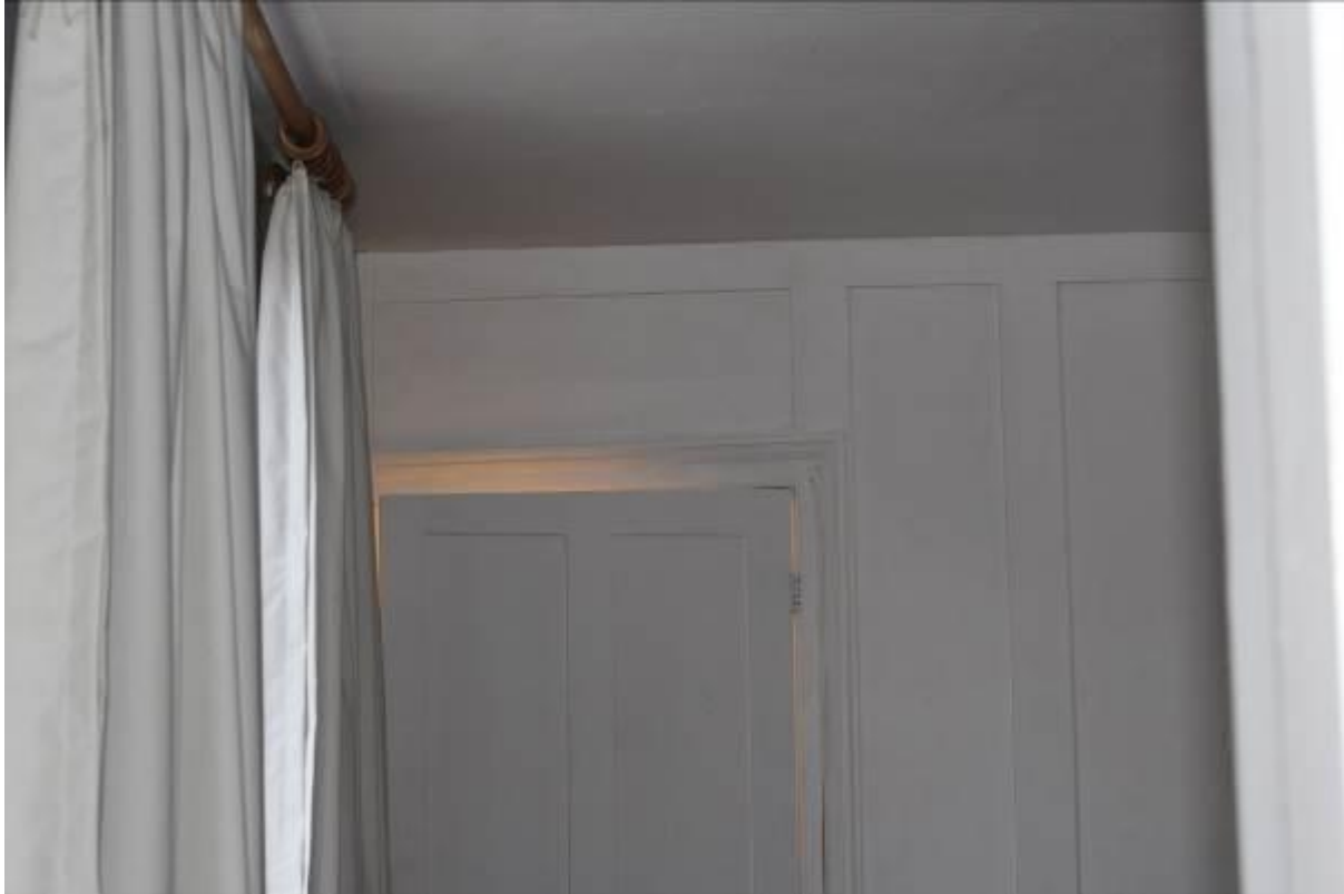
40. Door openings to the rear addition are out of alignment.
