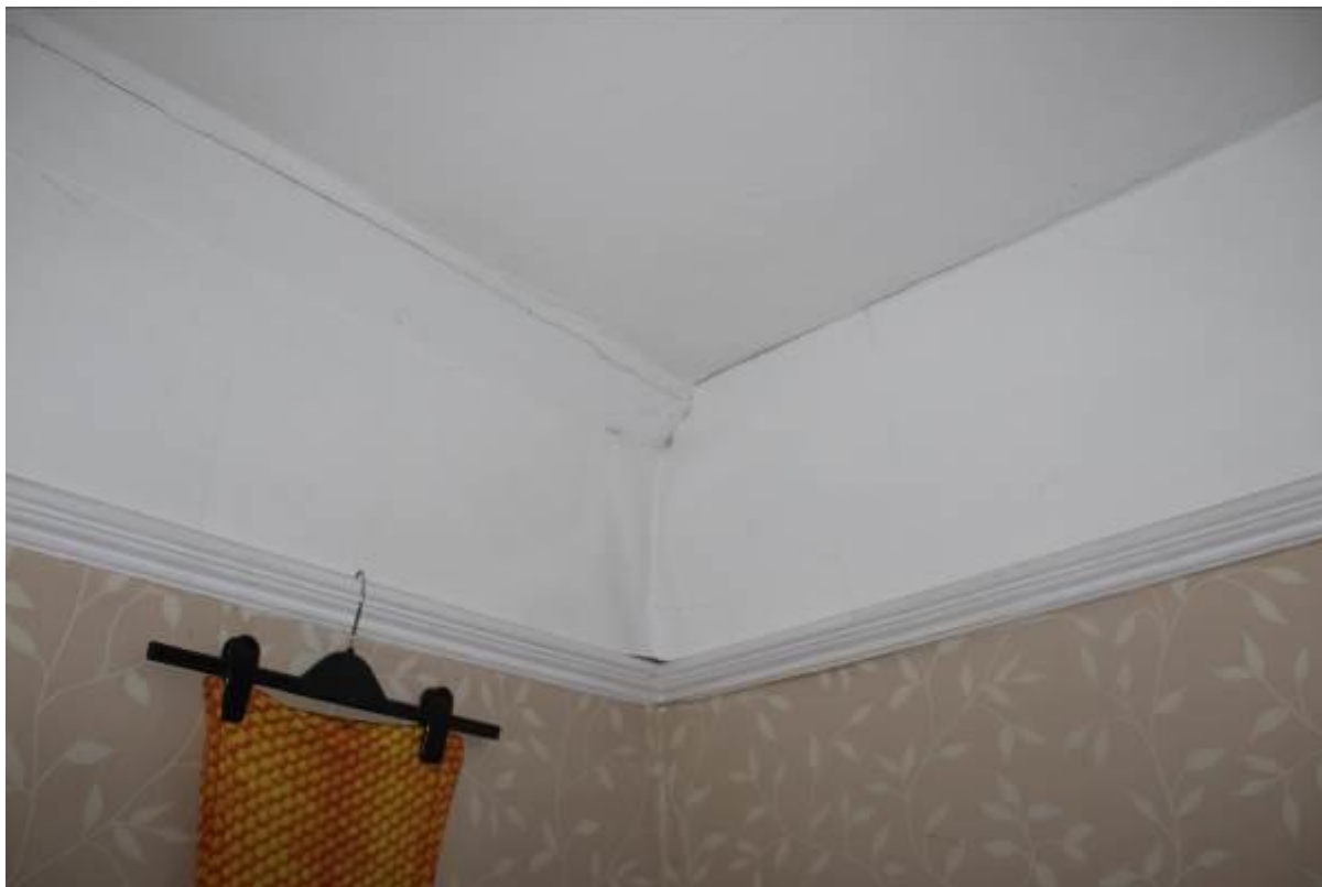
36. Some minor movement evident in first floor bedroom.
