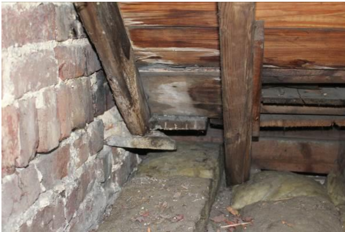
34. Support to base of rafter not ideal but currently satisfactory, this needs to be monitored or strengthened in some way.
