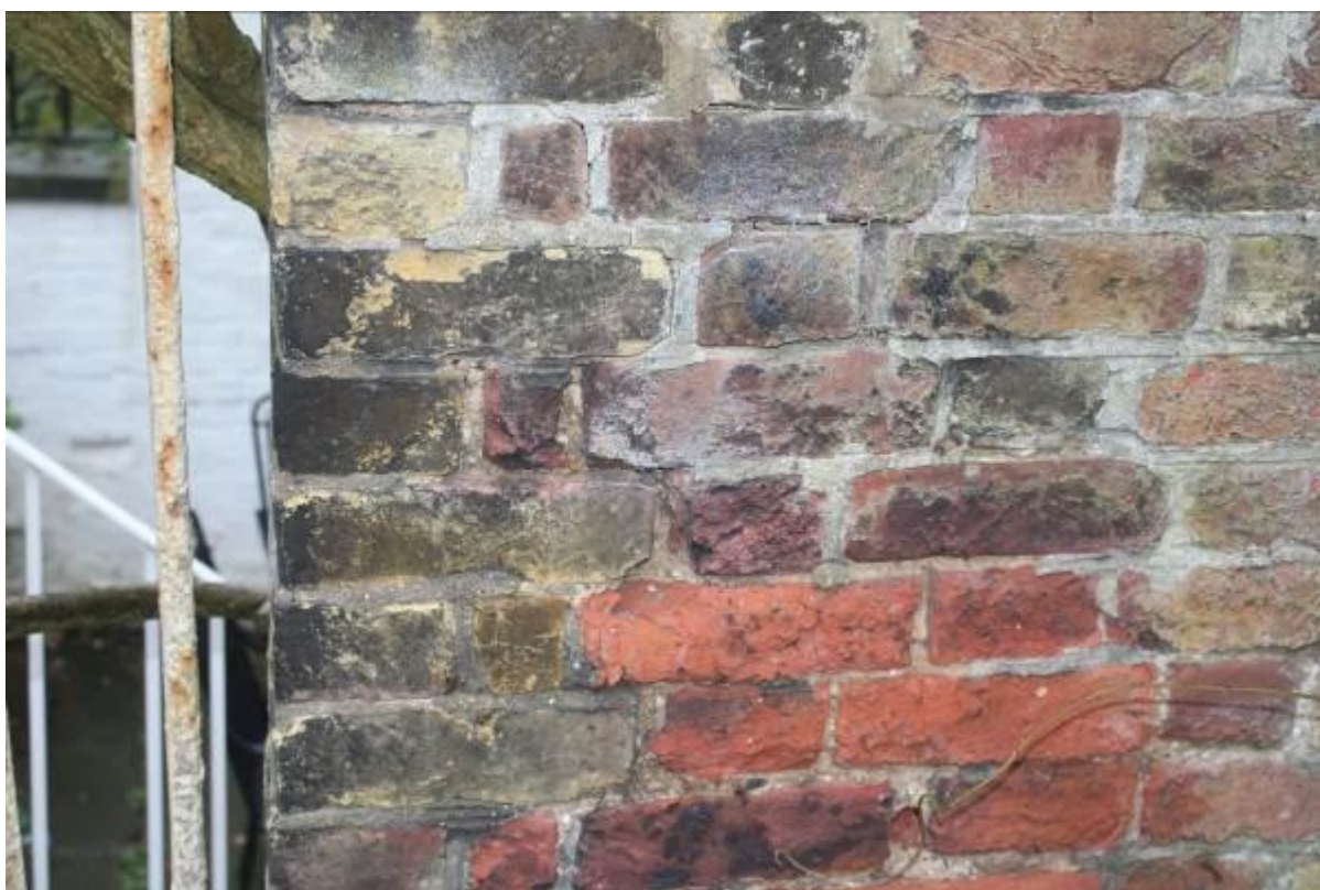
10. Some minor brick boundary repairs also required.
