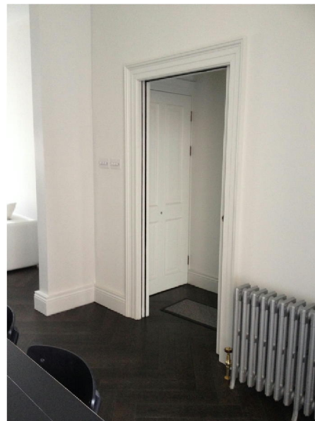
Ground Floor Living Room Views Left: Existing ground floor front chimney breast. Right: Ground floor doorway to the living room.
