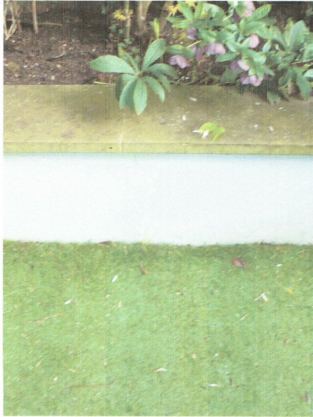
Cracking to adjacent retaining walls
