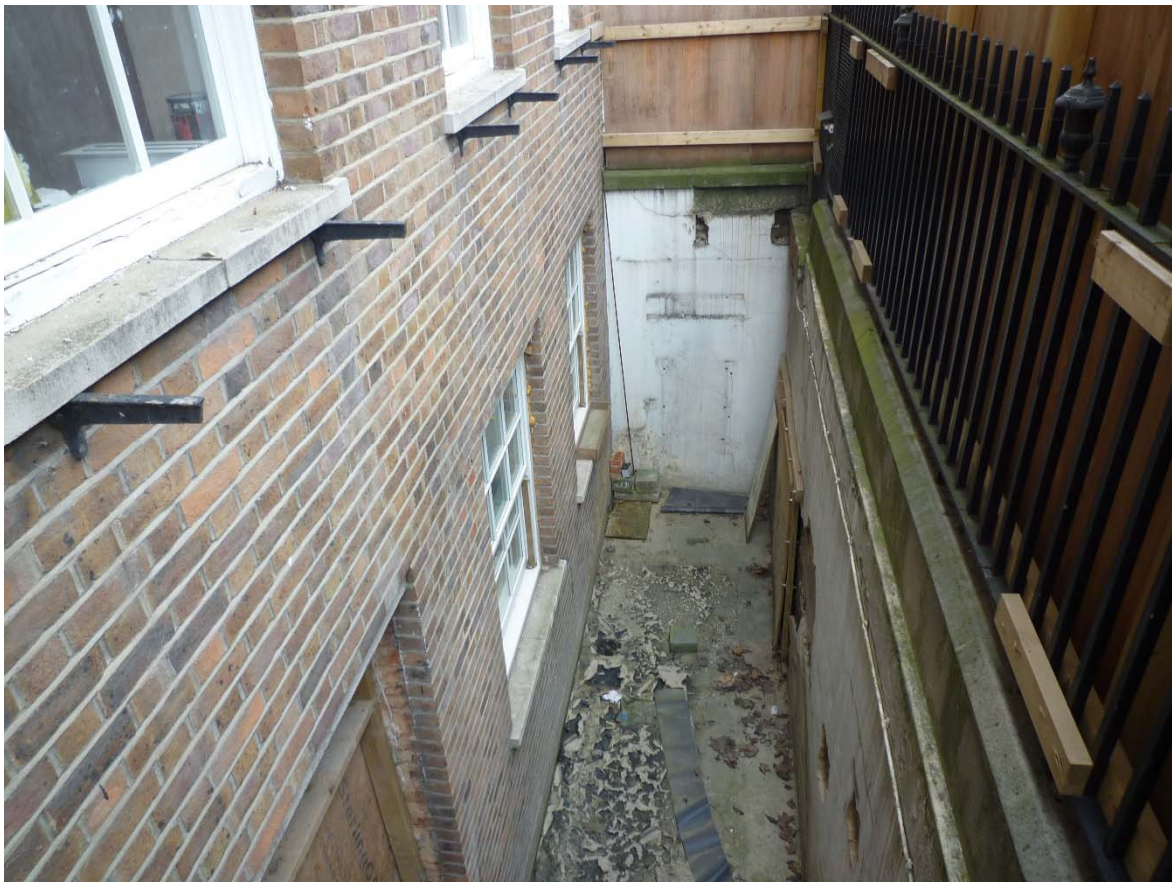
Fig.4 The front area, showing what may be the original 18 th century finials on the modern railings.
