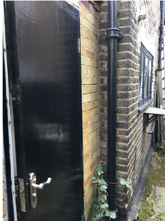
Figure 9 The west wall of the existing rear extension is set in from the side of the outrigger. It is proposed to move the extension wall outwards to make it continuous with the outrigger wall.
