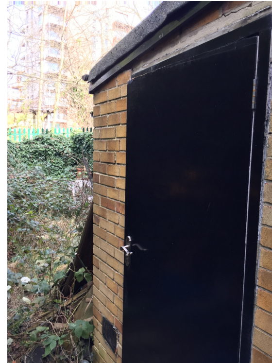
Figure 6 The shallow pitched roof and blank door do little to add to the character of the original property.
