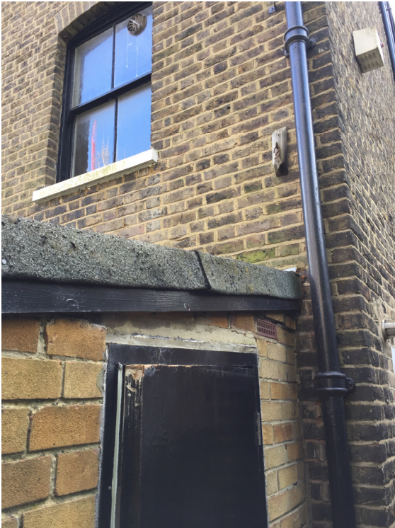
Figure 7 The existing roof to the rear extension is of a poor quality and detracts from the rear elevation of the original house.
