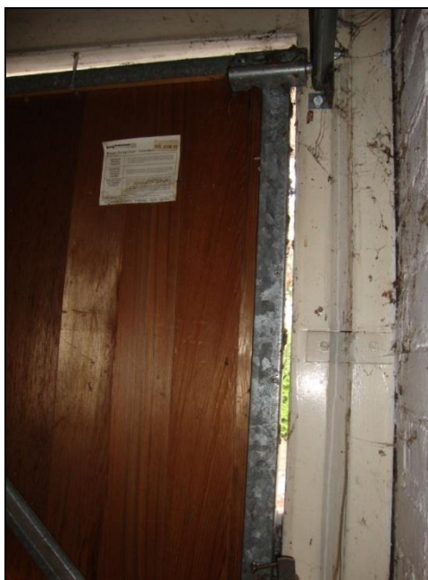
Photograph 1: Gaps surrounding the garage doors
