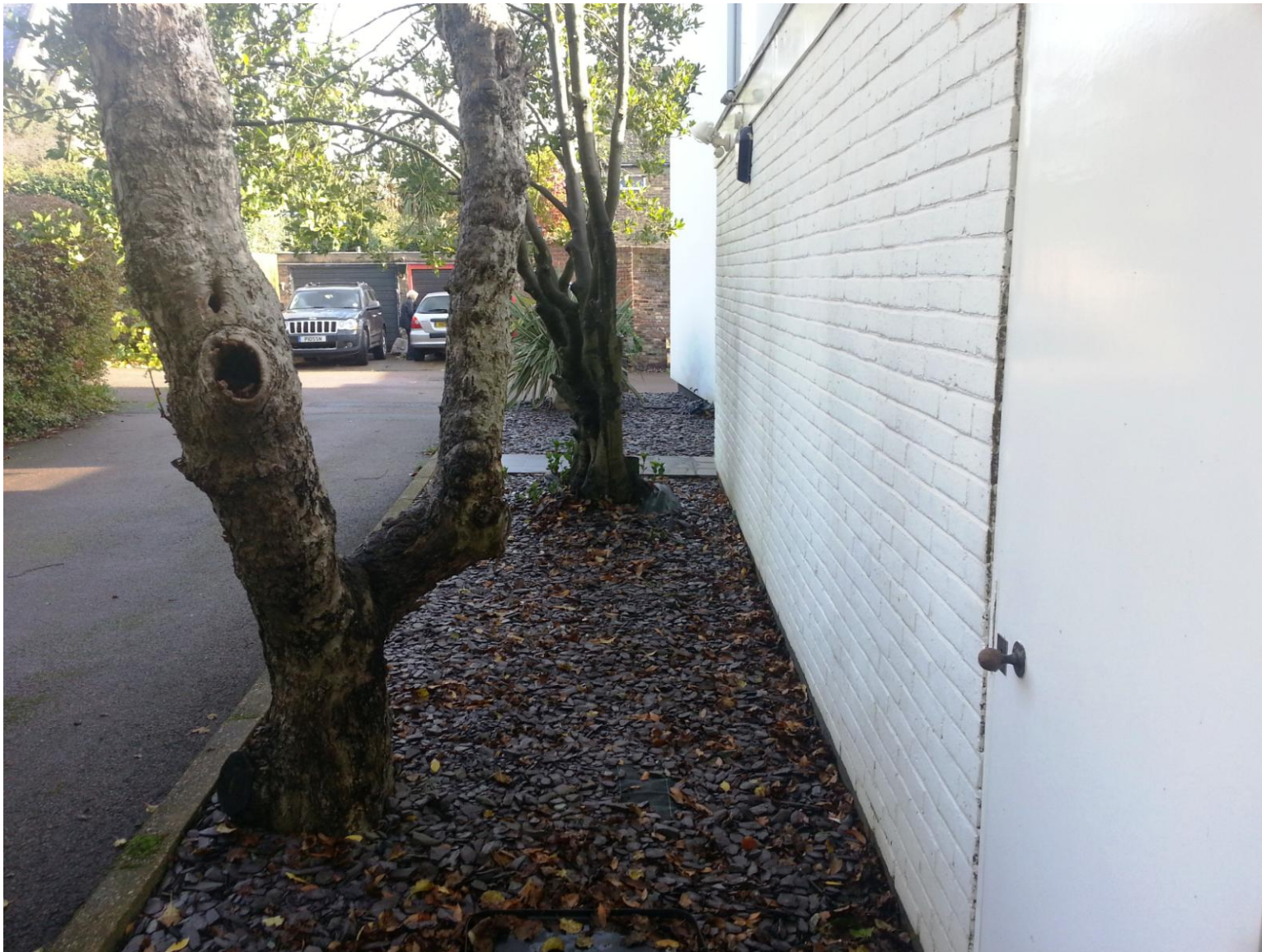
Close up showing proximity of trees T1 and T2 to the existing building
