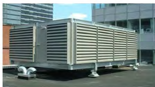
Louvres to new Plant Enclosure
