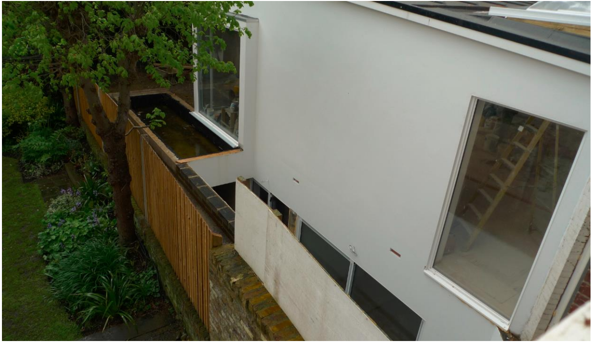
Photo 8: Existing unauthorised basement as part of 2012 scheme that was refused planning permission
