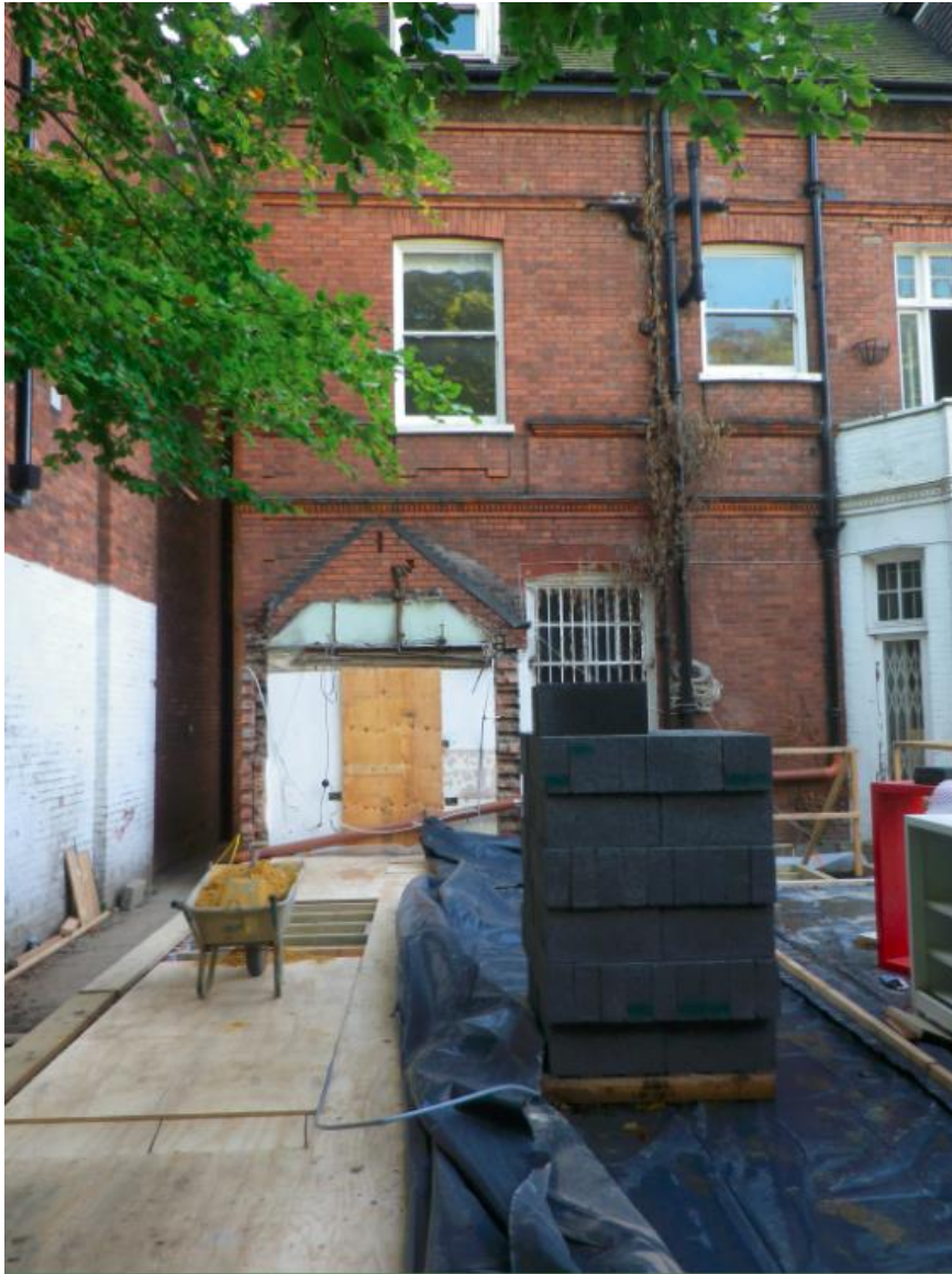
Photo 3: Rear elevation of the property following removal of the original single storey rear extension
