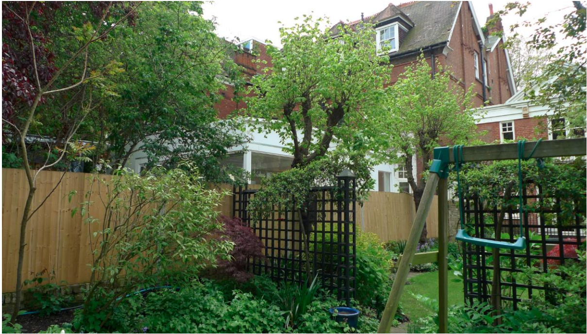
Photo 10: View of existing unauthorised single storey rear extension as part of 2012 scheme that was refused planning permission from garden of no. 43a Lancaster Grove
