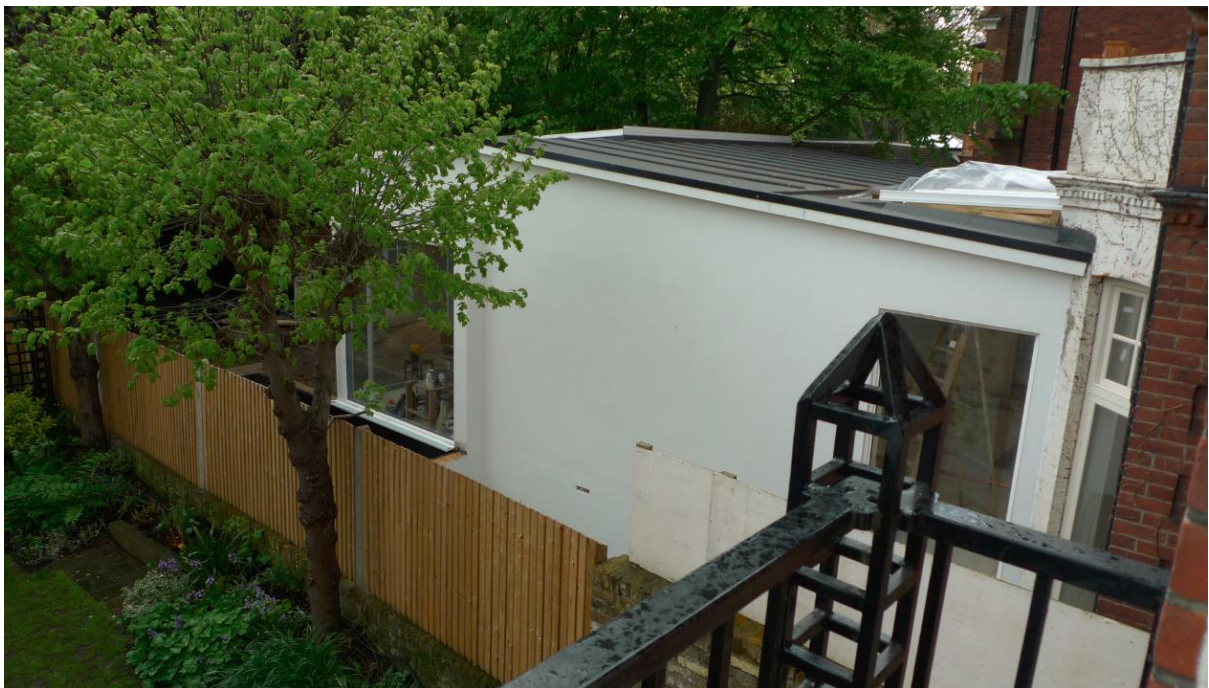
Photo 7: Existing unauthorised single storey rear extension as part of 2012 scheme that was refused planning permission
