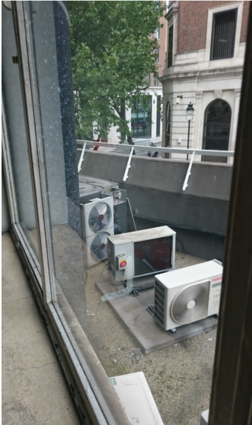
Photo 4: existing AC units at this level
