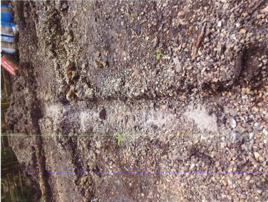
Pictures D & E. Previous foundation
