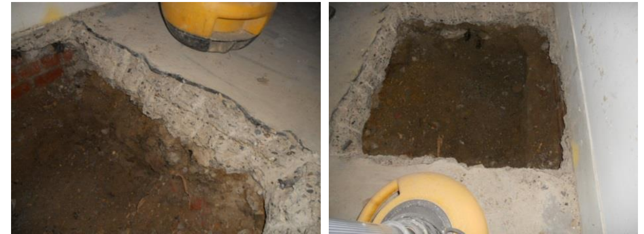
Figure 31: 2010 trial pit in Lower Ground Floor of No. 36 Chester Terrace shows non-original concrete slab and tanking.
