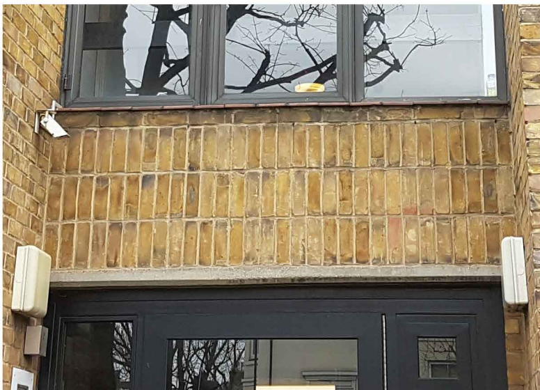
4. 254-256 Camden Road, Ashton Court; bands of soldier course brick between recessed door and window openings
