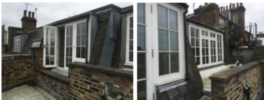
Figure 5. Grove End House, showing set back in existing mansard roof to accommodate a ‘means of escape’ route from the adjoining property.
