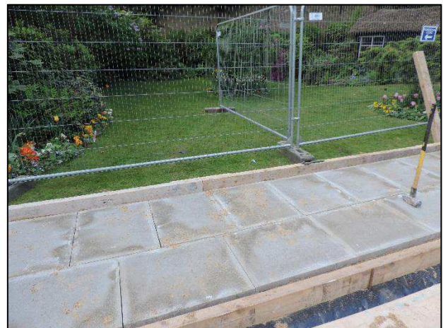
Photo 2: Area of completed slabs ready for the concrete to be poured. Heras tree protection fencing to the rear of the slabs.
