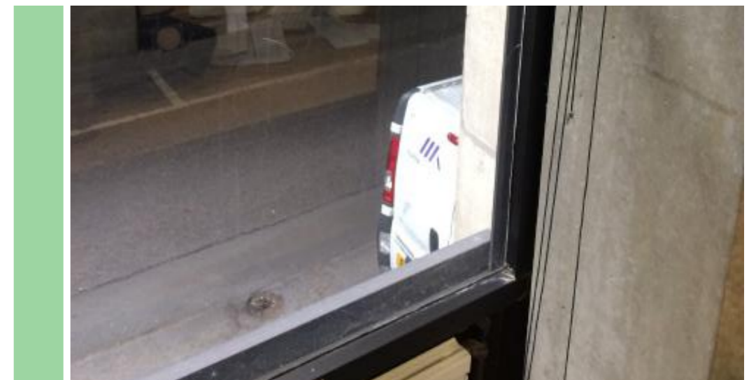
Photo showing no secondary glazing (New secondary glazing to be installed)
