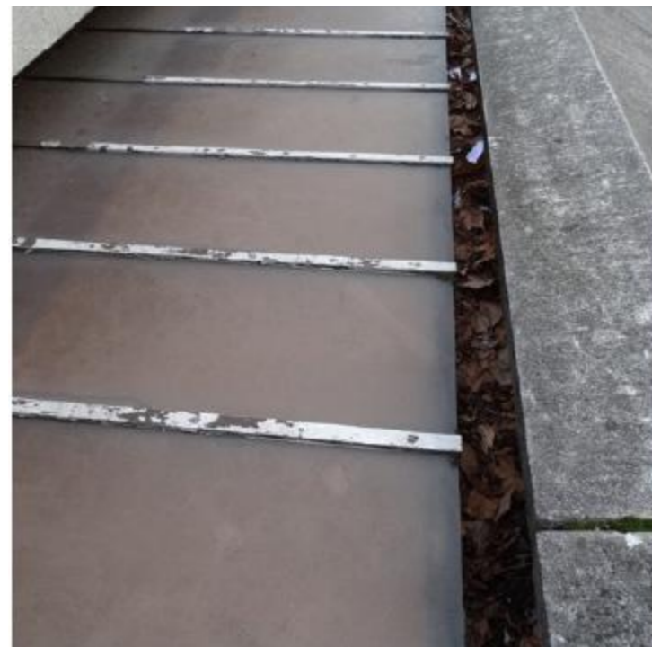
Wired glass rooflights on Level 3 wing to be replaced
