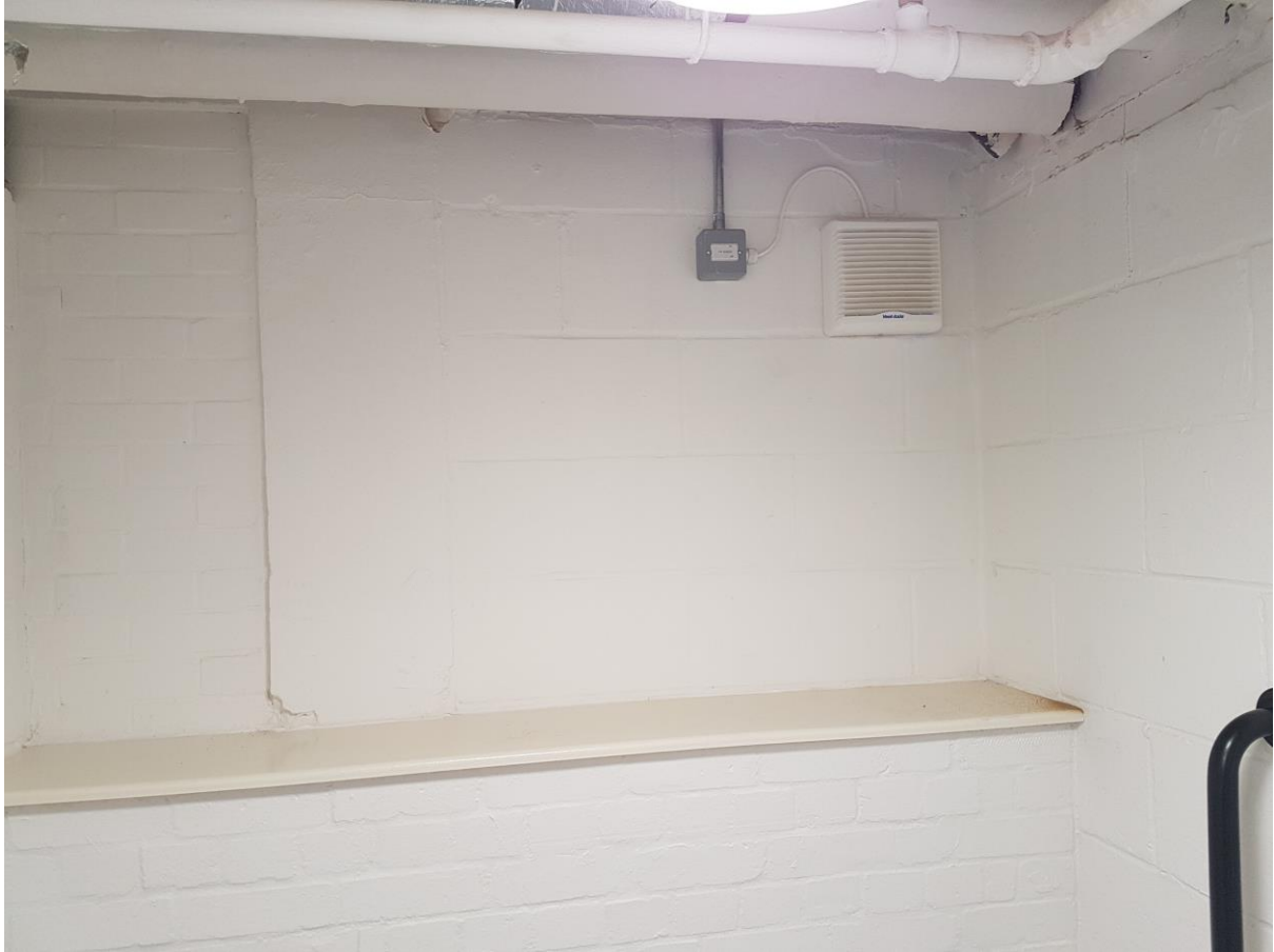
Current fan installed
