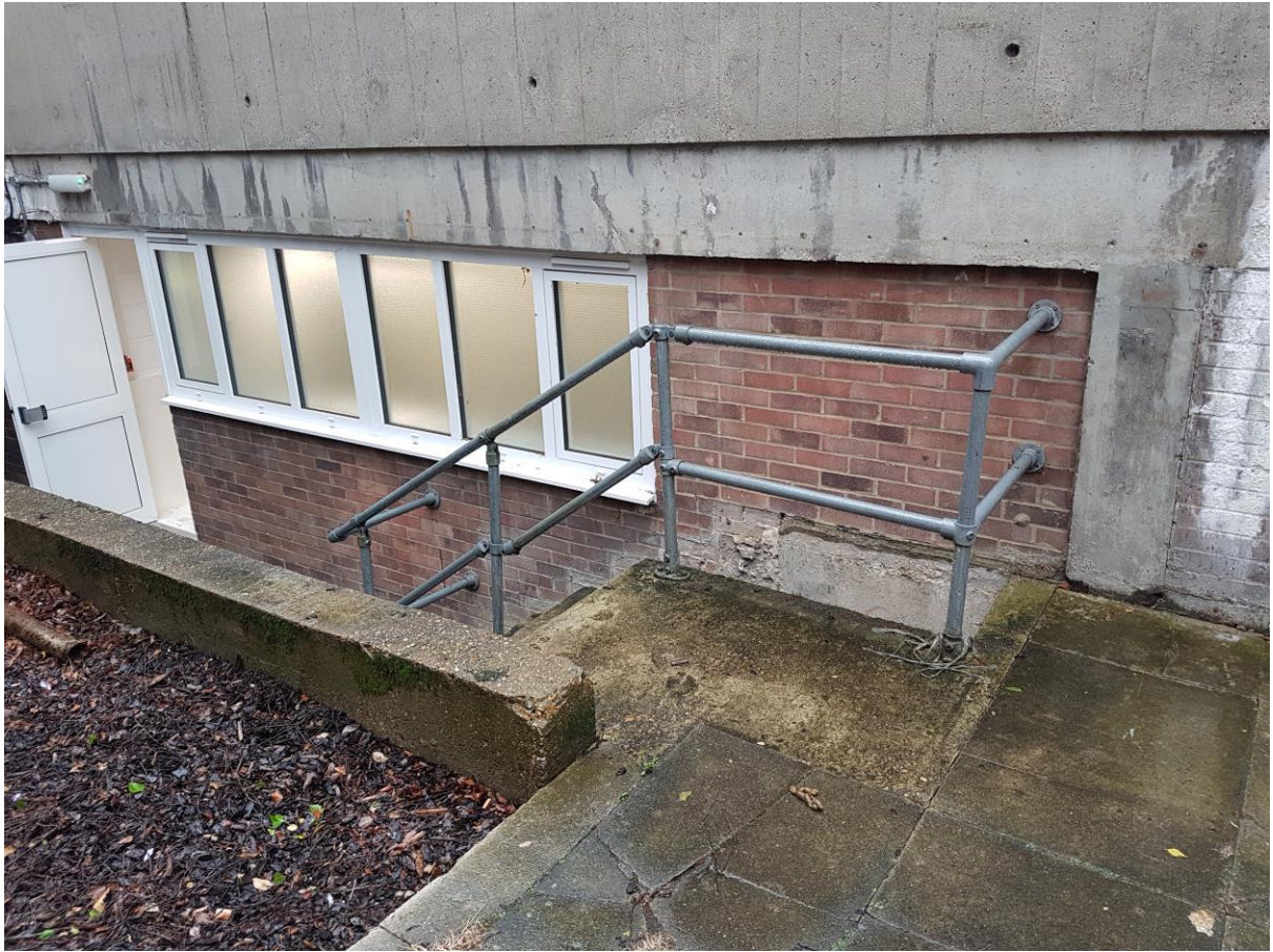
The fan exit of the fan will be on the bricks next to the window.
