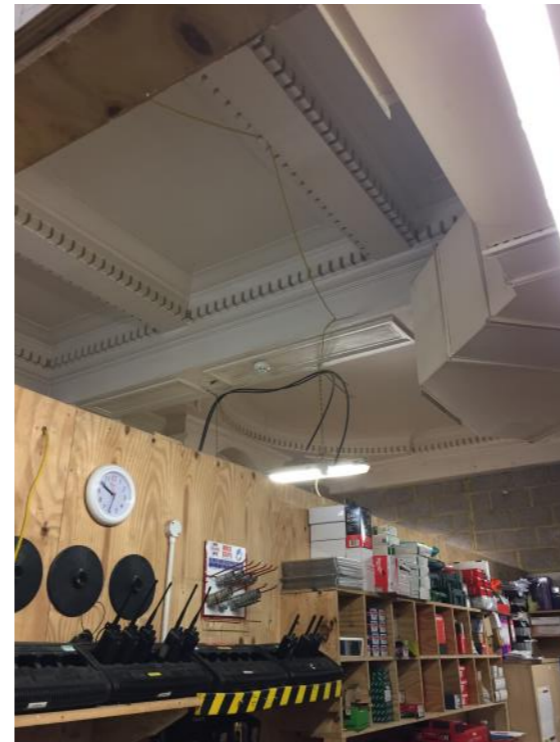
Plate 6: Ground Floor ceiling with replica down stand cornices and breeze block rear wall
