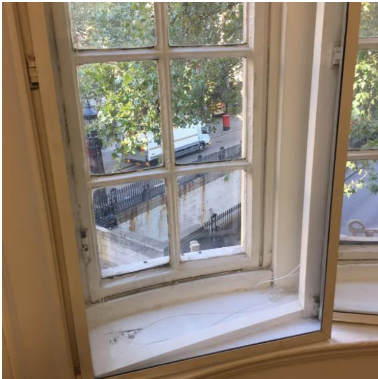
Plate 4: Windows with secondary glazing system in need of overhaul
