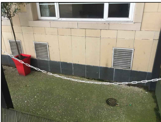
IMG007 OUTSIDE AIR LOUVRES TO RESTAURANT PERIMETER FAN COILS
