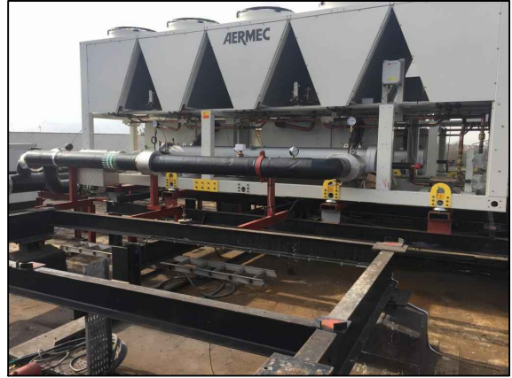
IMG002 NEW CHILLER; SPARE PLANT SPACE
