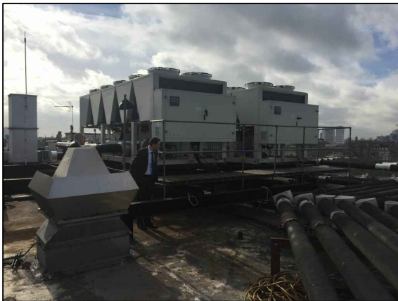
IMG003 VIEW OF CHILLERS + ADJACENT PLANT SPACE
