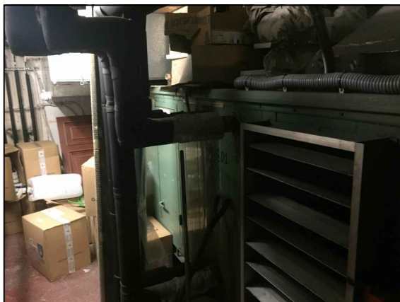
IMG005 EXISTING AHU PLANTROOM – NO SPARE SPACE
