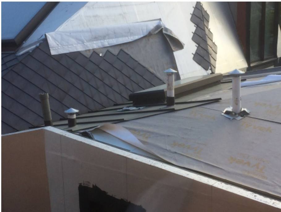
4. Examples of unfinished vent ducts viewed from side of 26 Belsize Lane
