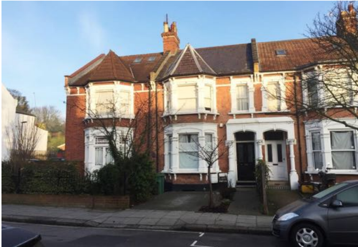
Photo 1: Front elevation (looking north-west). No.63 Hillfield Road is a part three-storey, part two-storey mid-terrace house arranged over split levels, with an original cellar. (Photo courtesy of Vorbild Architecture)
