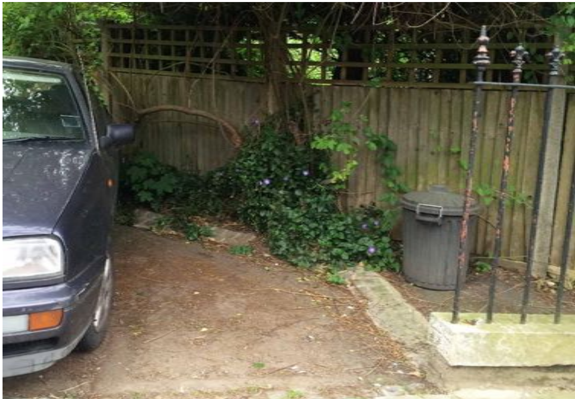
Photo 6 (below): The rear boundary to No.63's rear garden consists of a wooden fence with concrete king posts and wooden gravel boards. In front of the fence is a short ramp, formed of granite setts.
