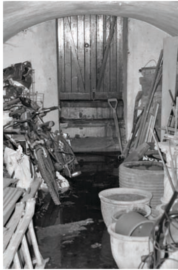
Photo 2: Flooded Vault 4 and garden tools.
