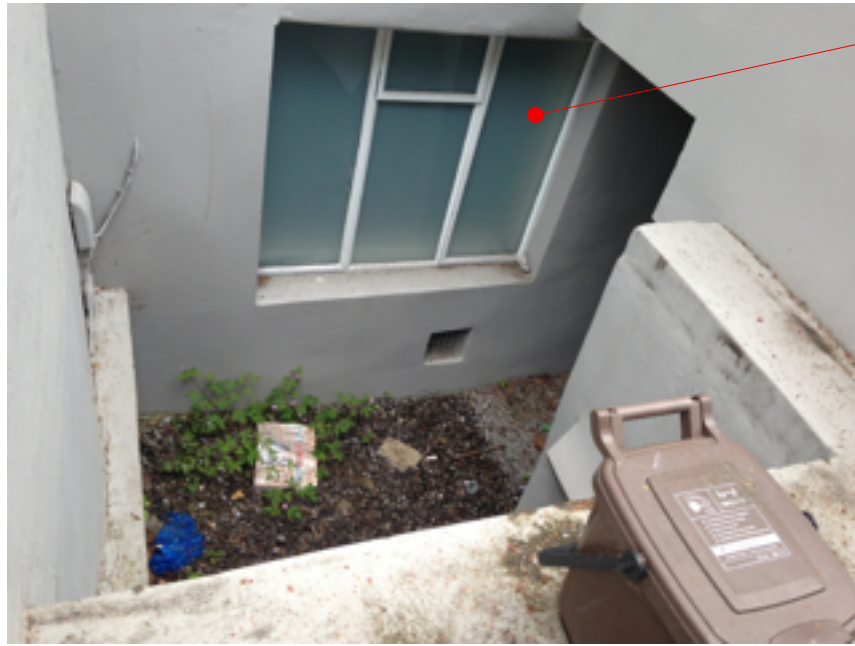
LG-W01 LIGHTWELL WINDOW EXISTING TO BE REPLACED
