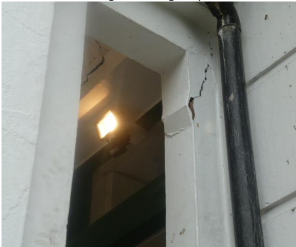
Rotation cracking to storm porch
