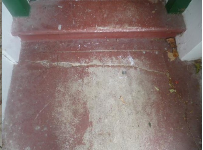
Cracking to storm porch floor
