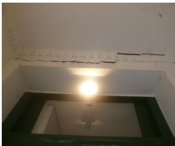
Cracking in storm porch
