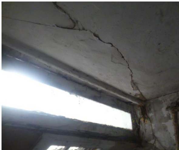
Cracking in garden flat below porch
