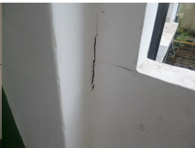
Cracking in storm porch
