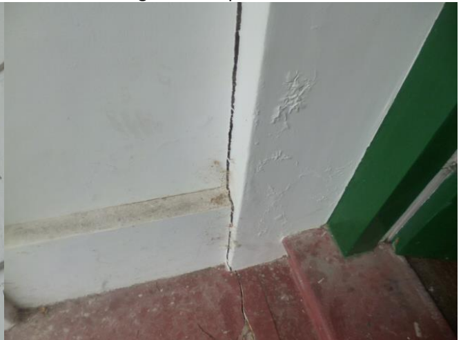
Cracking to left wall in storm porch
