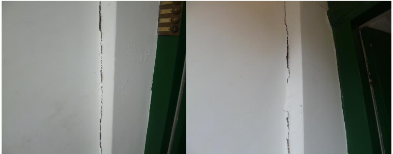
Cracking in storm porch
