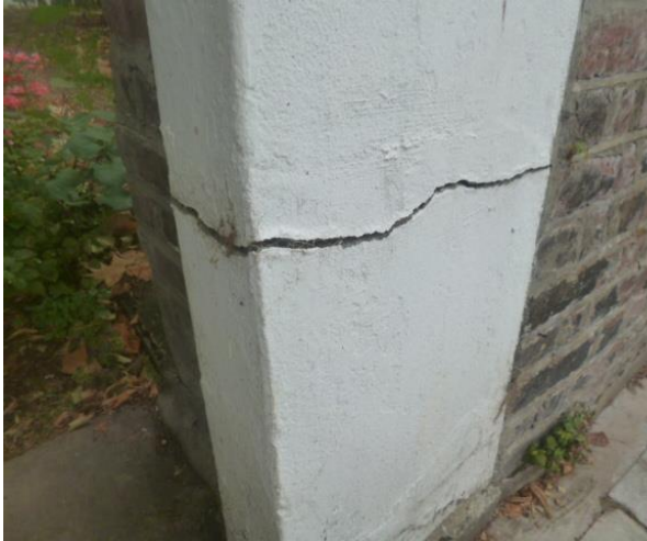
Cracking to front gate pier
