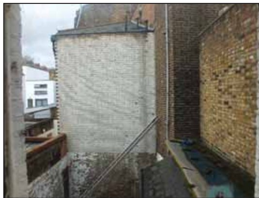
Photo 9: View from the rear window of No.110 into the area to be developed, looking west
