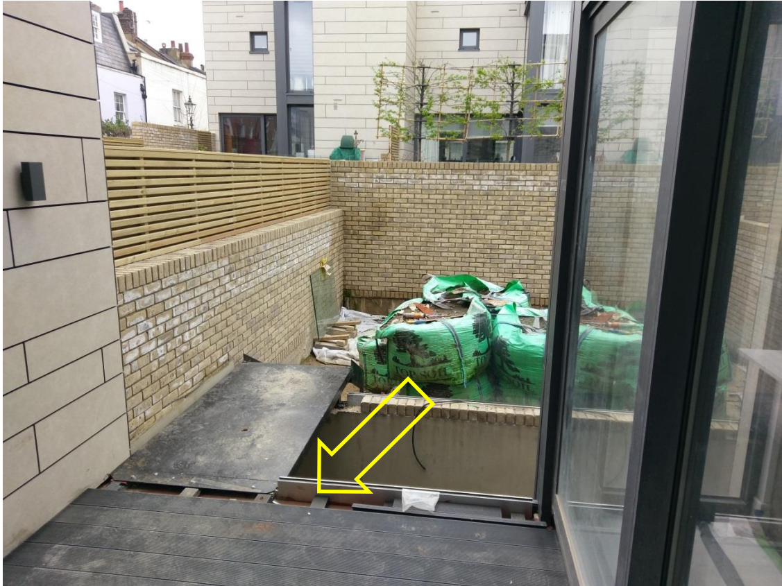
Photo.1 View from within No.10 looking west towards parallel block. Arrow indicates extent of proposed extension.
