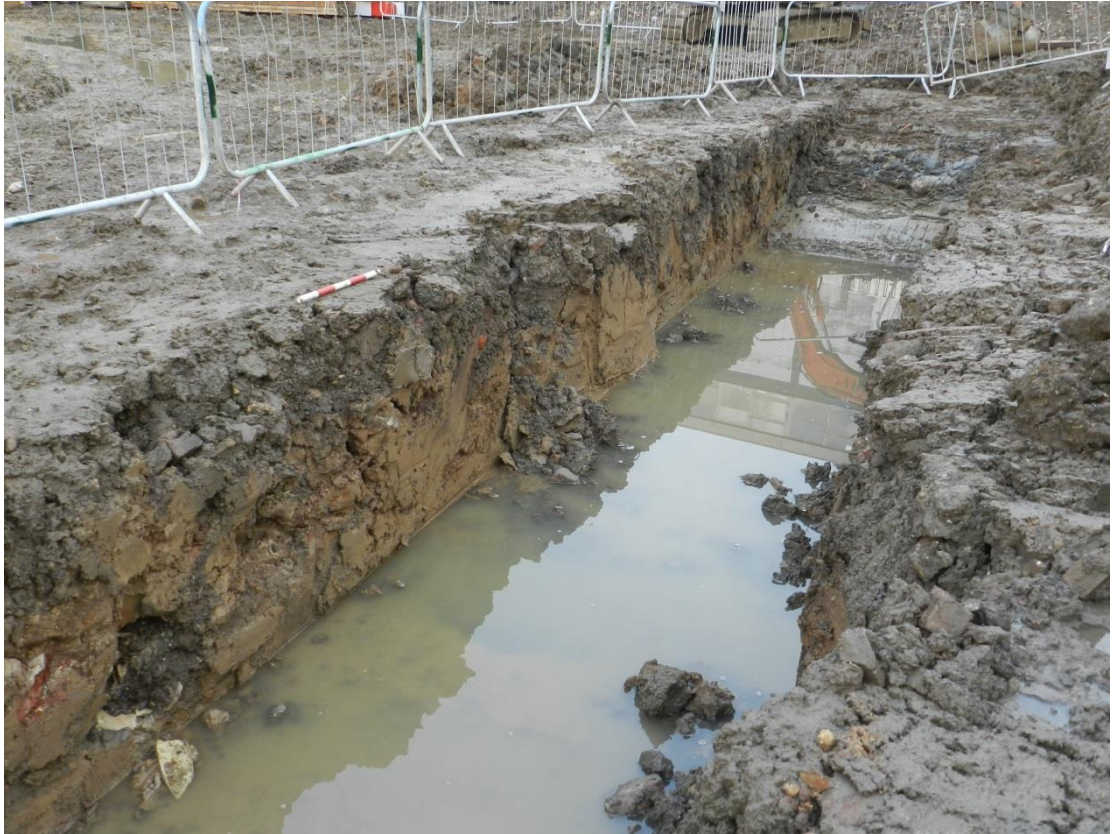
TR2 looking north showing east-facing section with made-ground overlying London clay and a ceramic water pipe in the left foreground.
