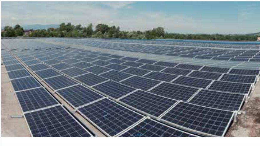
Slovenia Installation: 150 kW | S-Dome System
