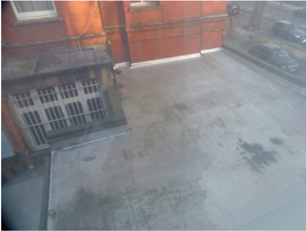
Photograph of the flat roof of the link between both building that will be split along the line of the Party Wall
