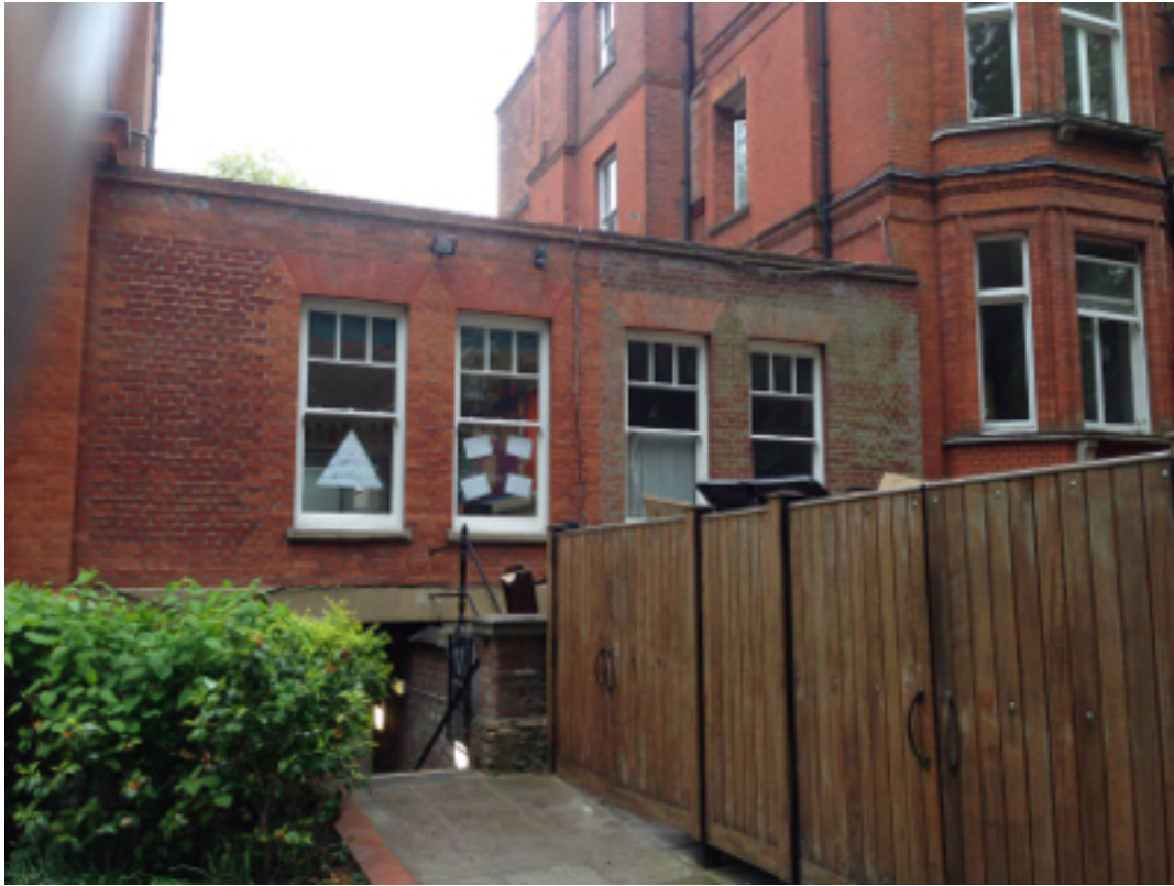
Photograph of the single storey link to be retained from 47 Fitzjohn's Avenue.
