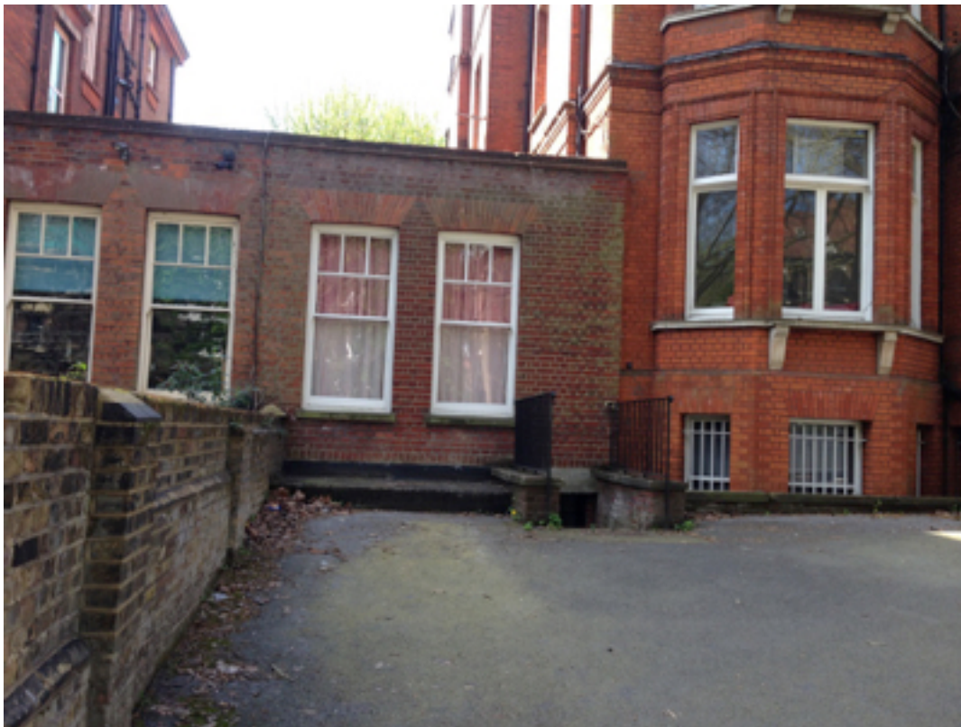
Photograph of the single storey link to be removed from 49 Fitzjohn's Avenue.
