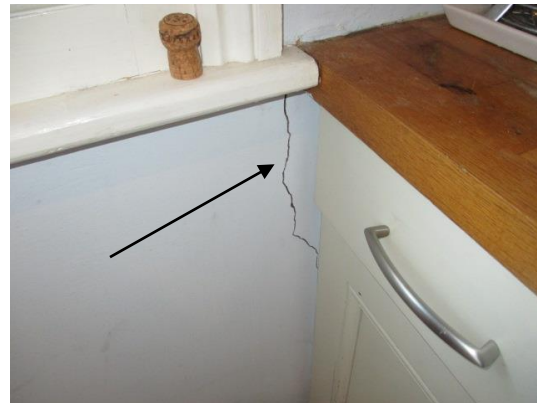
Cracking in ground floor flat kitchen
