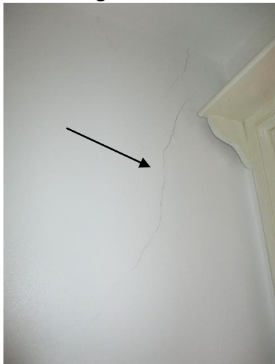
Cracking in ground floor flat hallway
