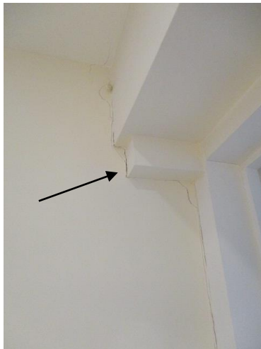
Cracking in upper flat stairway at rear addition junction
