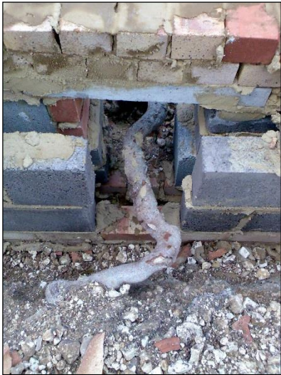
Examples of a constructed brickwork Void-Former surrounding a root in excess of 50mmØ.
