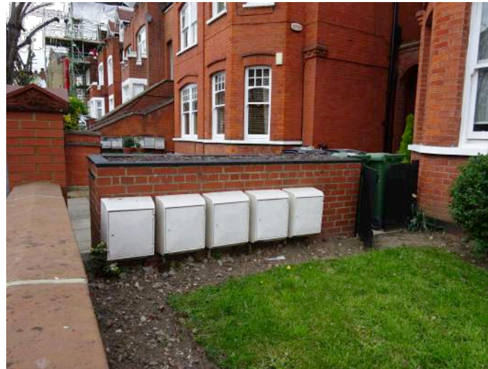
Existing Gas meters - to be retained as existing
