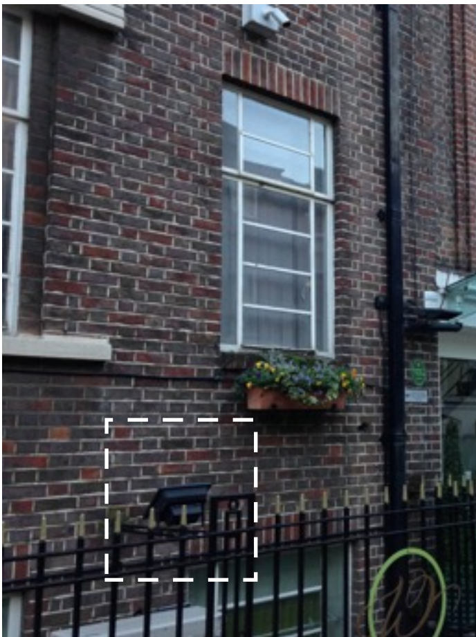
Unconsented facade floodlights on Euston Street railings ( 14 ). Proposed to be retained.
