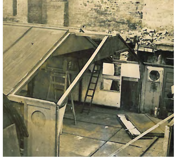
The two huts under construction, they were erected with the efforts of 'Old Bedfordians', ex-Bedford School Boys.
