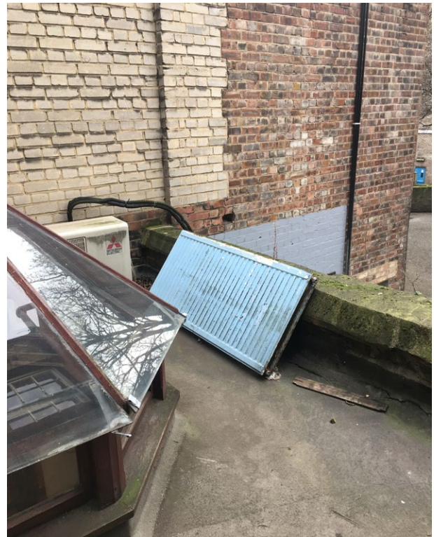
The existing lantern rooflight is in a poor state of repair and often leaks into the restaurant below.
