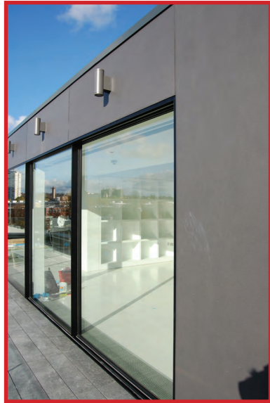
Grey fibre cement rainscreen cladding panels to match existing on 4th floor.
