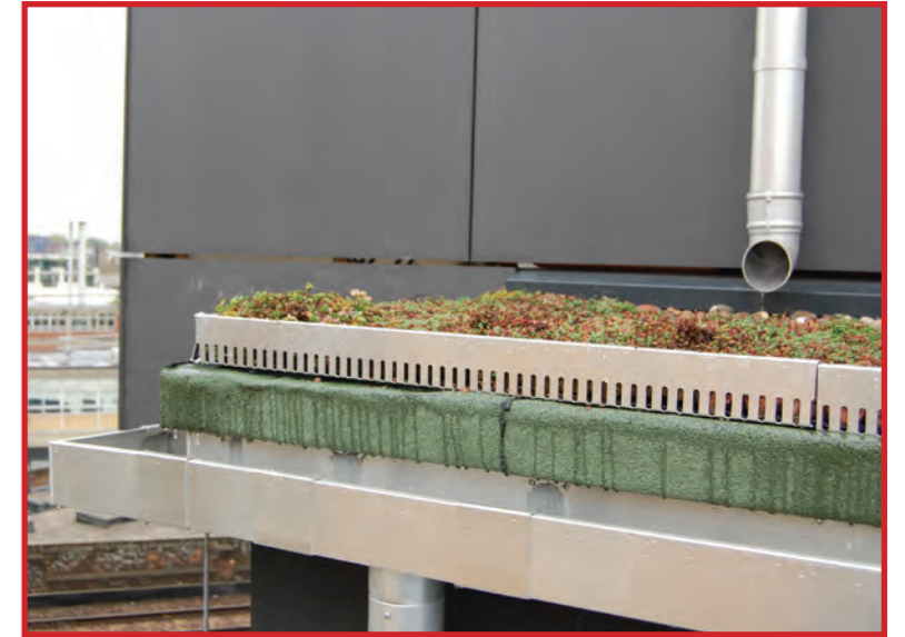
Sedum blankets planted on new roof, with aluminium rainwater goods to match existing. All visible rainwater goods kept off of street elevations, as per existing.
