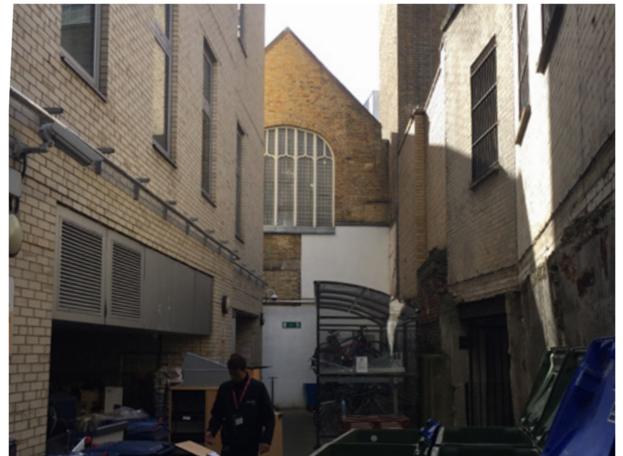
View of the space between Aviation House and the hall. This elevation remains unchanged. The lower level of the hall is occupied by changing and shower facilities.
