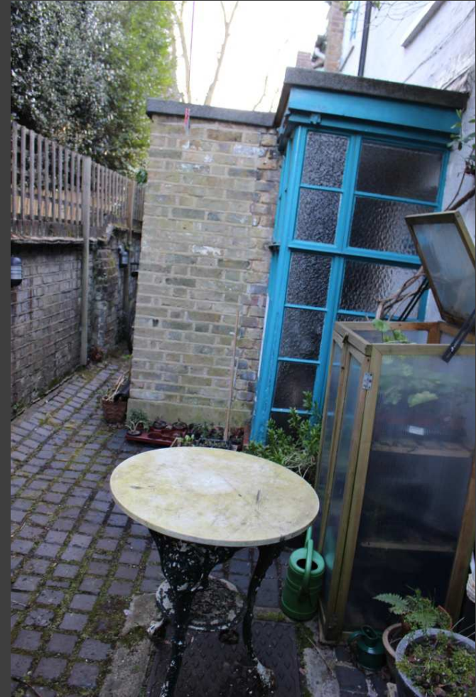
View of rear single story extension showing steel window, WG.03 and existing flat roof.
