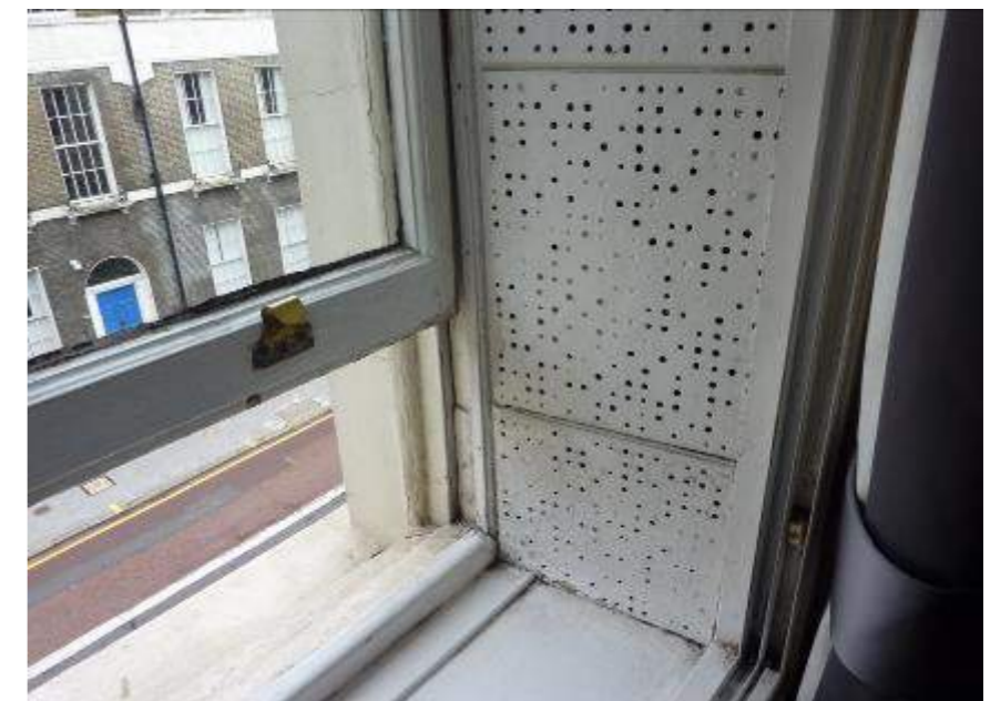
Figure 29: The historic installation of secondary glazing has had a detrimental side effect in the installation of unattractive perforated sound proofing where the original shutters were once located
