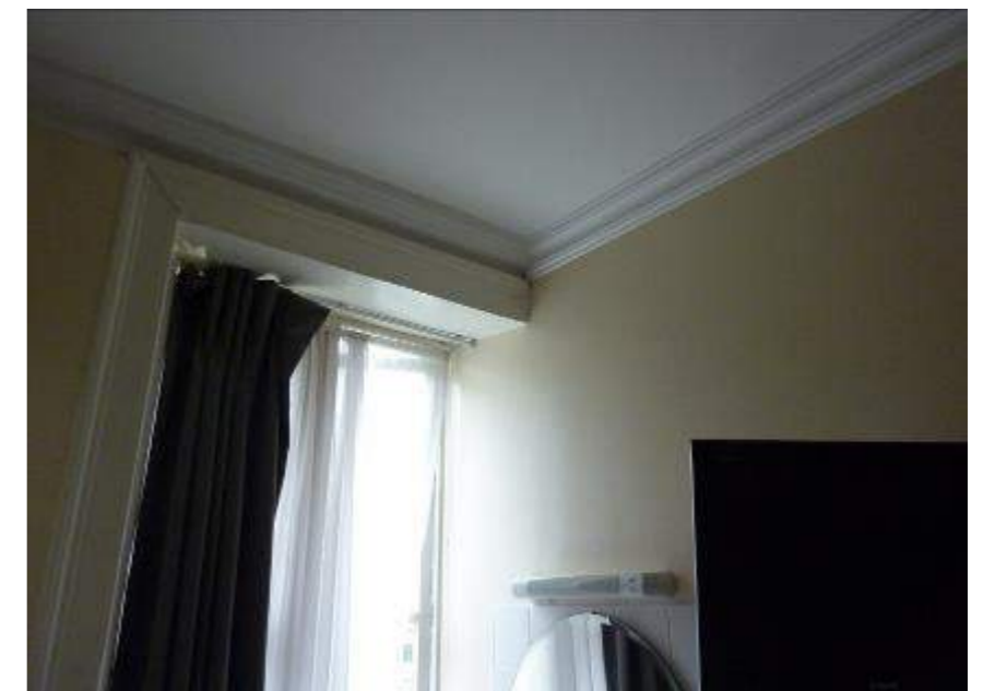
Figure 25: In a number of locations partitions have been insensitively installed - here blocking the window to No. 77, further eroding the building's special interest
