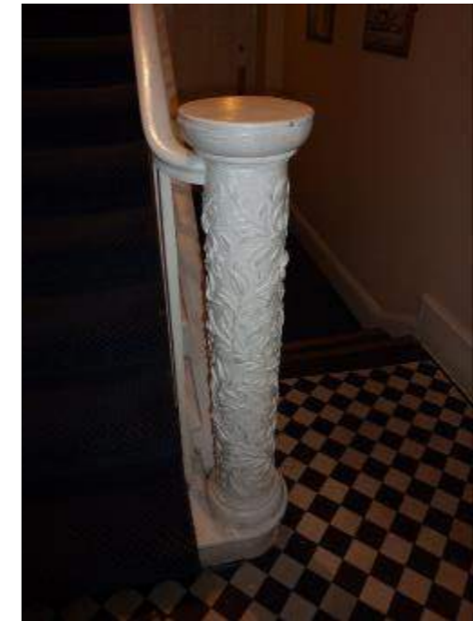
Figure 32: No. 79's ground floor newel post has been inappropriately altered with this clumsy foliage clad element
