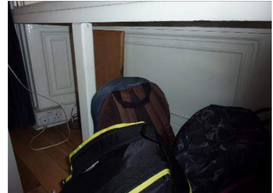
Figure 28: Original timber aprons survive below a number of windows
