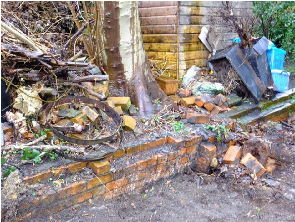
Image 9 Base of T6, showing level change and potential destabilisation once wall removed
