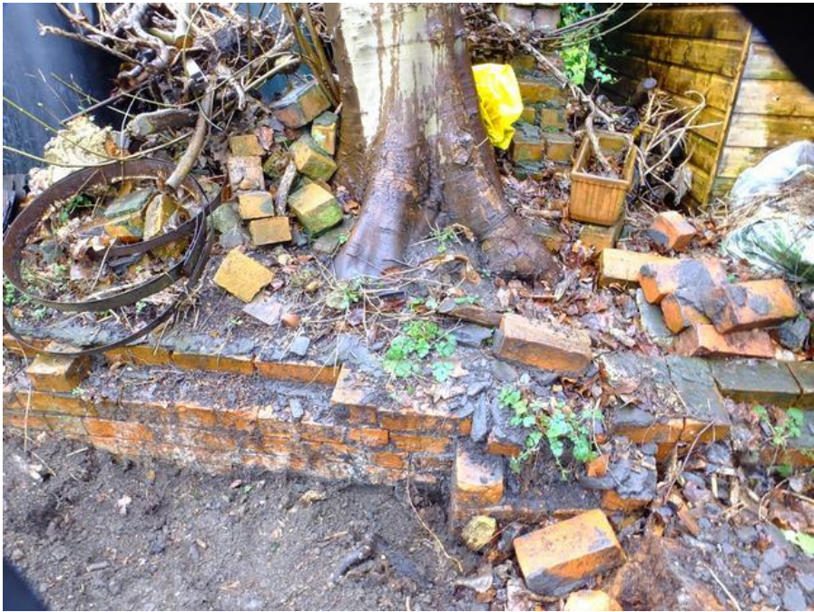
Image 10 Base of T6, showing level change and potential destabilisation once wall removed
