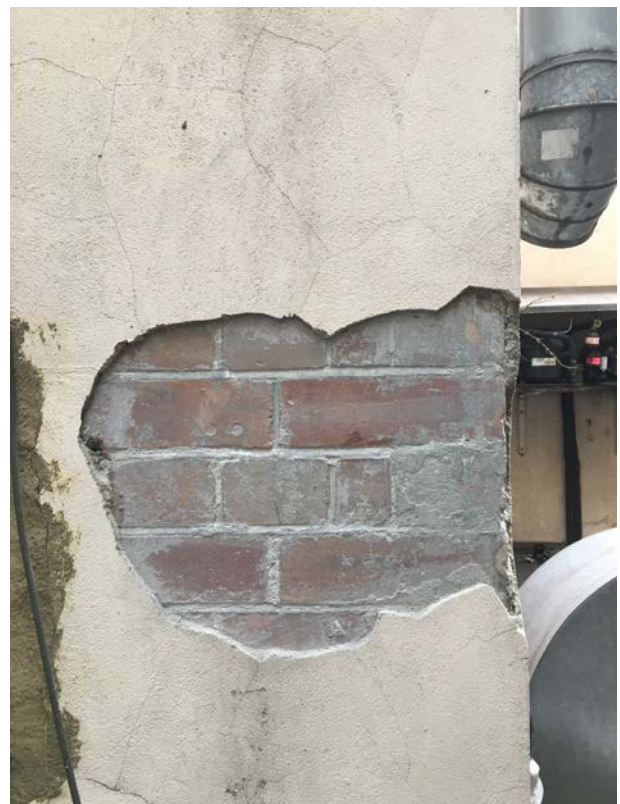
Trial exposing original brickwork which appears of high-quality and in good condition
