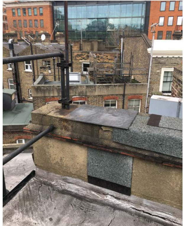
Cracked roof membrane to be replaced and coping repaired
