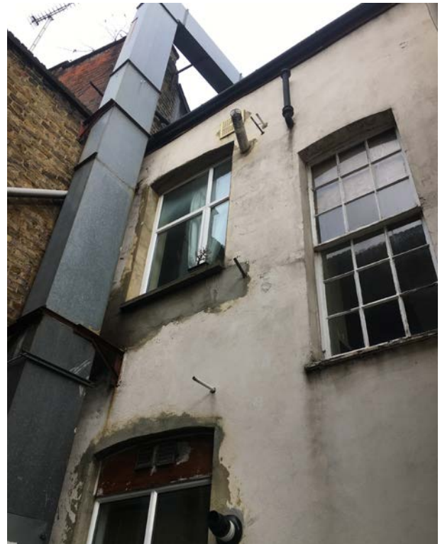
Poorly repaired and maintained render, untidy services and large extract duct
