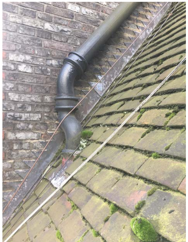
Tiles to be sensitively cleaned and vegetation removed
