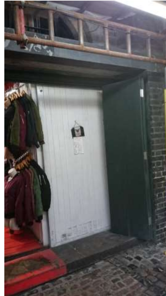
Figure 11: Chalk Farm Building, unit 32: individual sliding doors lie behind recently installed bi-fold timber doors which carry across both sub-units (January 2017).
