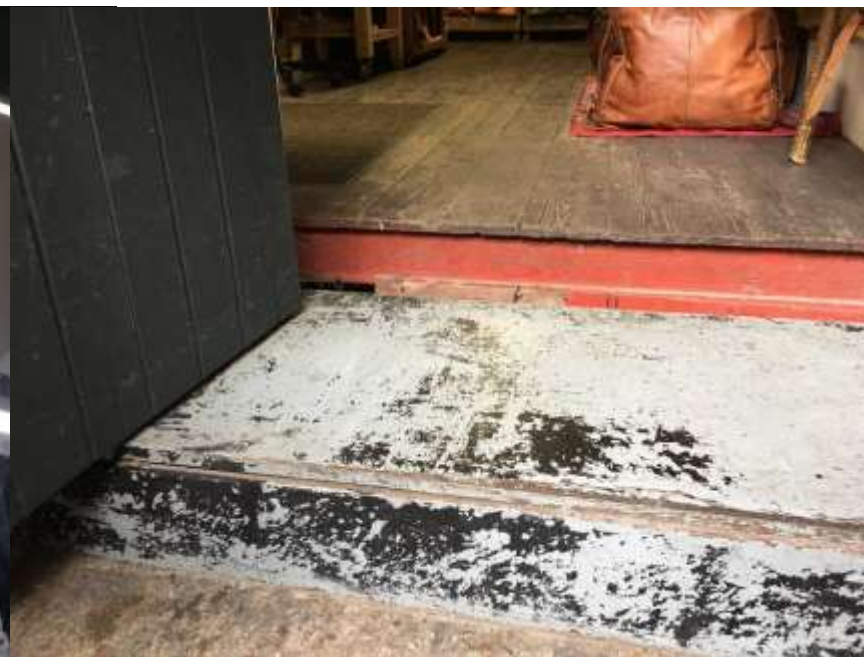
Figure 13: Chalk Farm Building, unit 29: makeshift timber steps currently serve each unit (February 2017).
