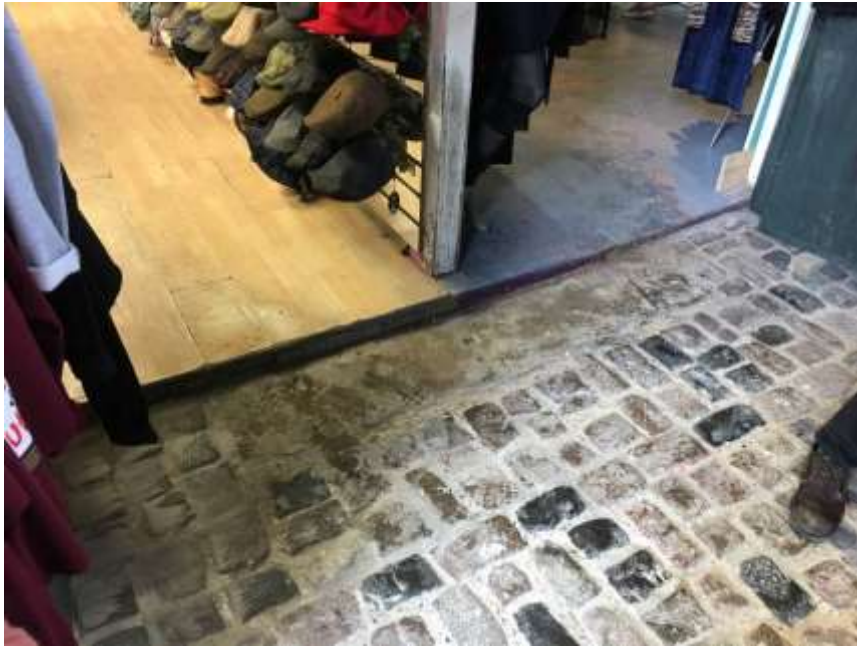
Figure 14: Chalk Farm Building, unit 34: In some units, floor finishes have been applied directly on top of a sloping concrete base (February 2017).
