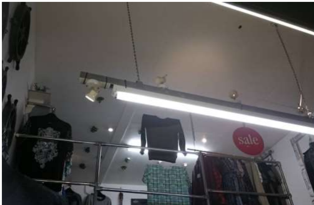
Figure 12: Chalk Farm Building, unit 31: view of the current wall linings existing in some of the units (January 2017).
