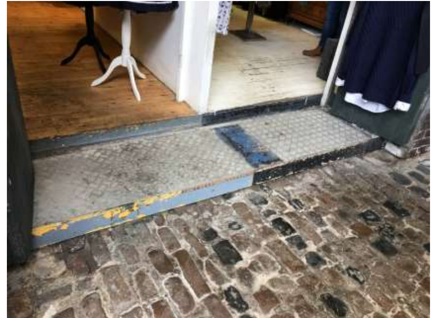
Figure 15: Chalk Farm Building, unit 31: In other units, the floor level is raised, with floor boards on battens with a brick substrate below.
