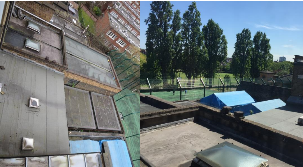
Photos showing the varied nature of the existing terrace and range of poor and ad hoc rear extensions.
