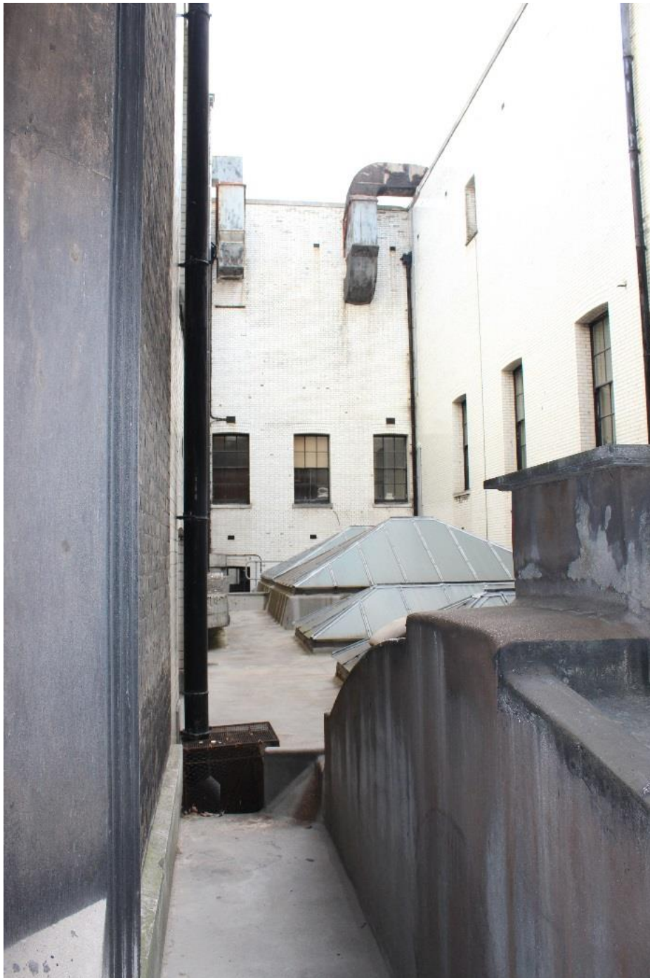
View of ductwork serving Galleries 43-45
