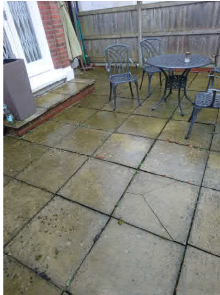
Photo 12 – Settlement and damage to rear paving
